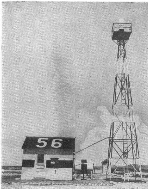
Figure 2.—Rotating beacon installation.
