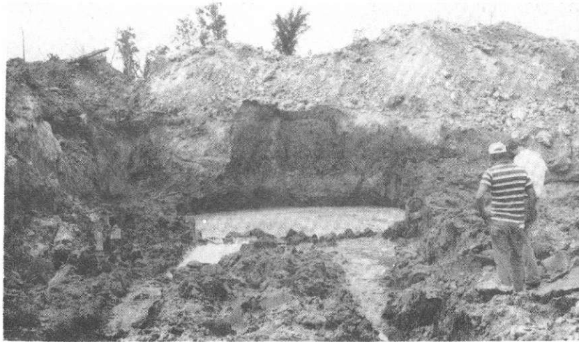
Figure A3. North wall of excavation. A pit about 50 x 150 feet was excavated to a depth of about 10 feet. A smaller pit, about 25 x 25 feet was then excavated to a depth of about 35 to 40 feet with a large backhoe. Water rose rapidly to the level shown (about 12 feet below surface) when the backhoe reached a depth of about 20 feet. Organic layer visible just above water level.
