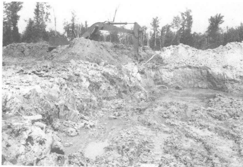
Figure A6. West wall of pit. Backhoe capable of reaching depths of 35 to 40 feet seen on left. Two pumps were used to lower the water table, but they could lower the water table only to a depth of 17 or 18 feet.
