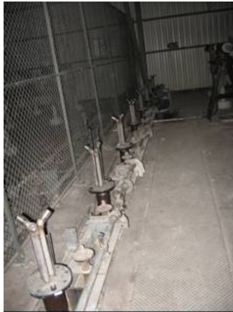
Figure 2-6. Toxecon™ II Lances Installed - View from ESP Roof
