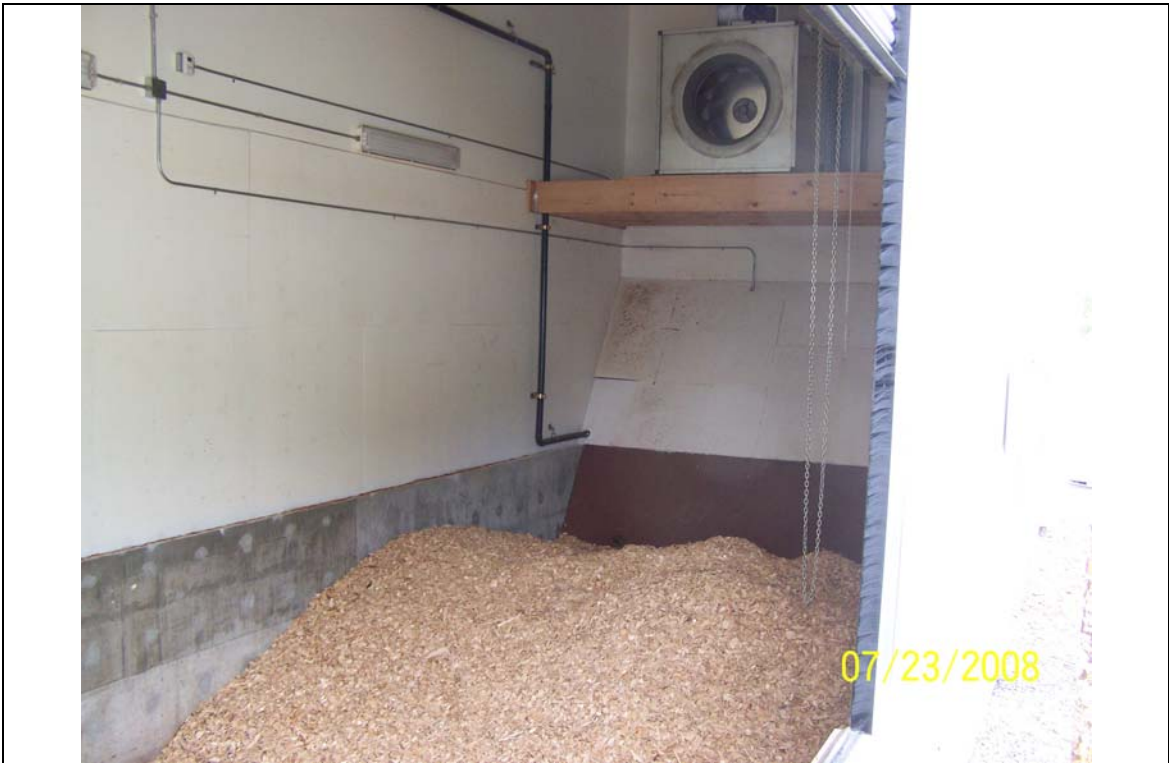
Wood storage bin loaded with chips. Note gable end exhaust fan above
