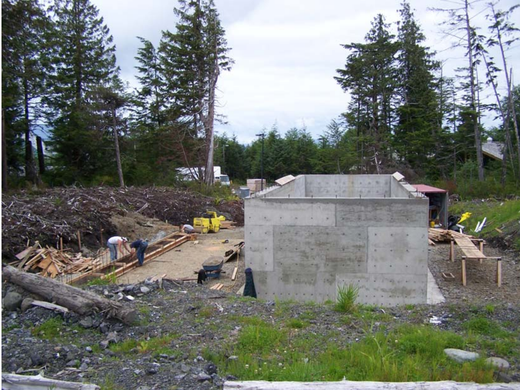
View of boiler building south wall. Wood storage area at right. August 2007
