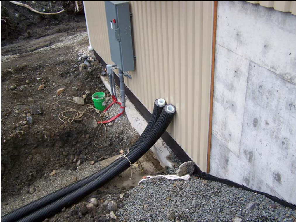
Hot water supply and return lines at pool south wall. January 2008
