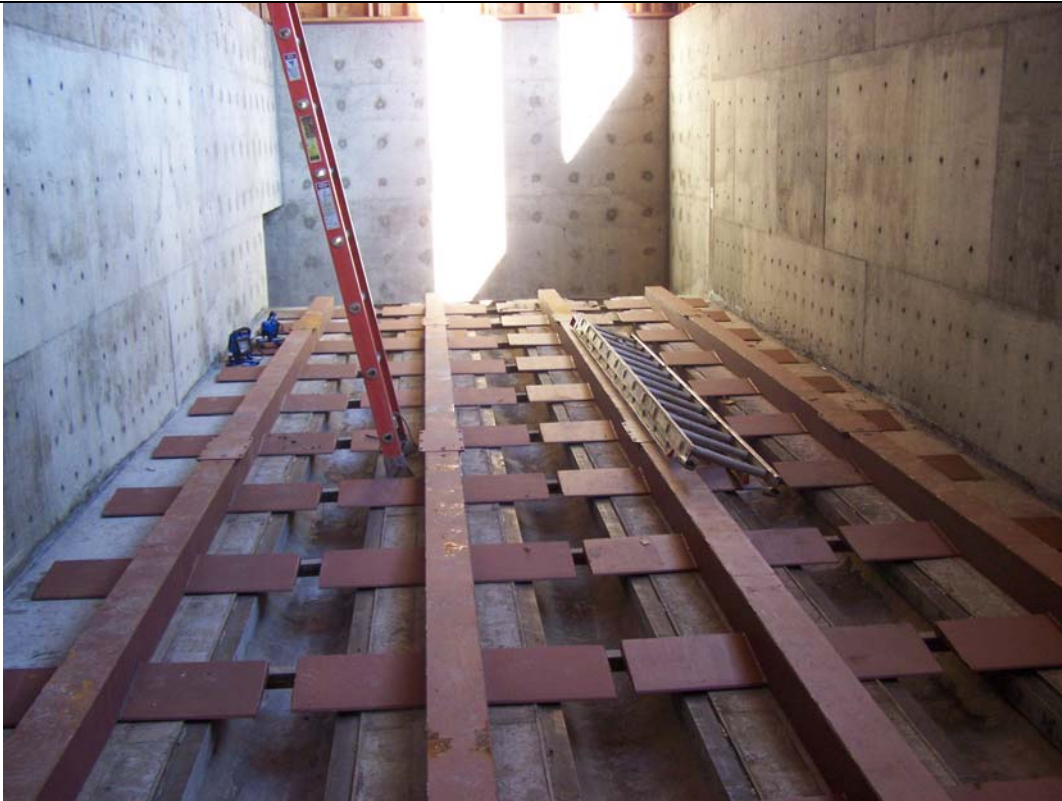
Wood storage bin floor. Note ram assemblies and air ducts. October 2007.
