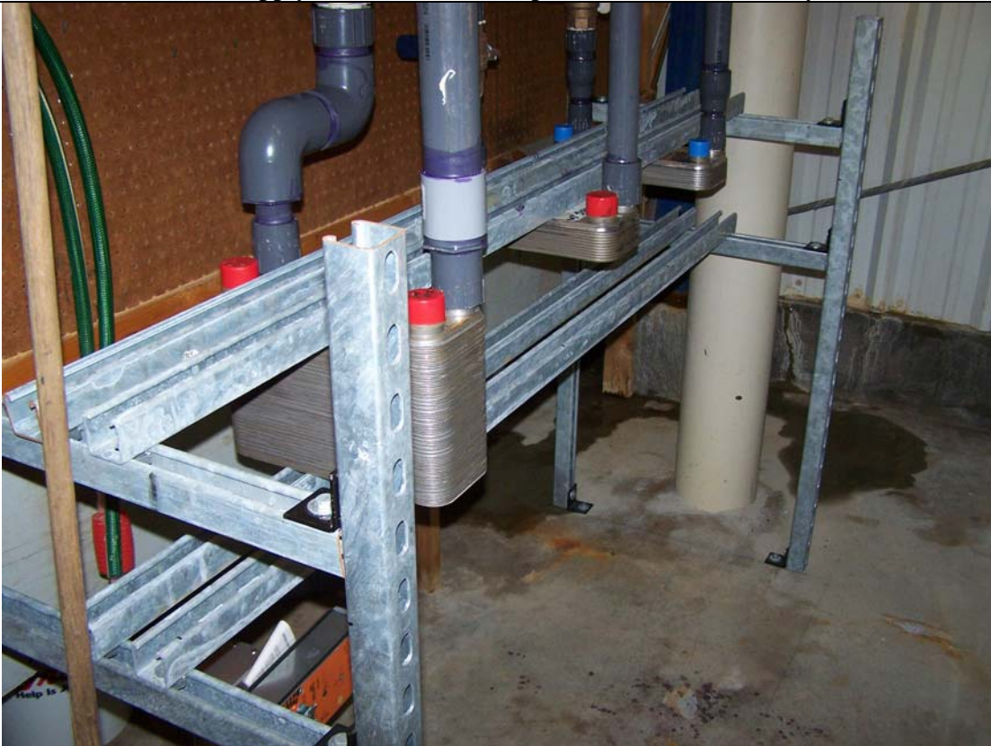
Heat exchangers at pool mechanical room. January 2008
