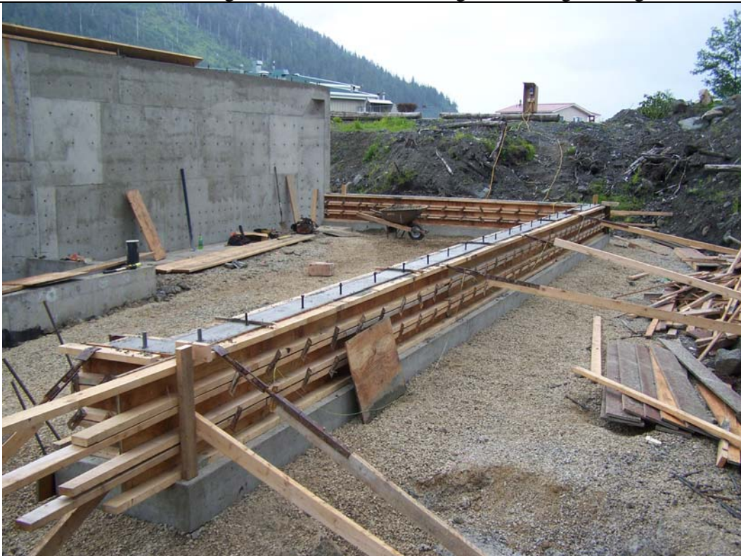
View of boiler building footing and stem wall at mechanical room. August 2007
