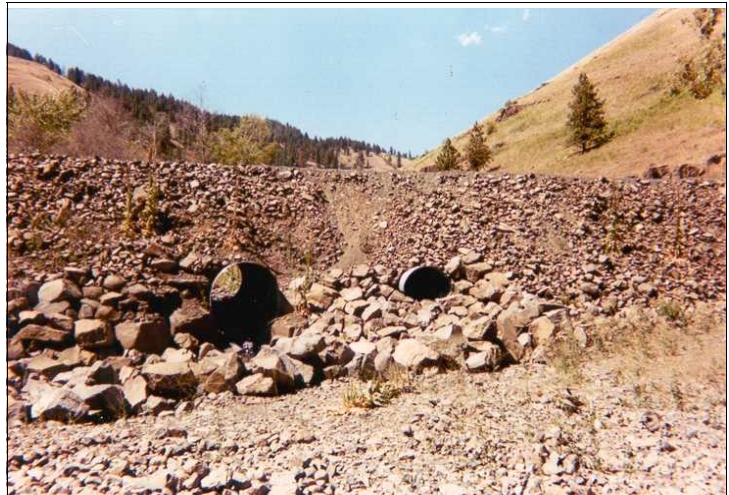
Pre-project: Grouse Creek, looking downstream at County Road with 2 culverts. Photo from Anderson Perry & Assoc.
