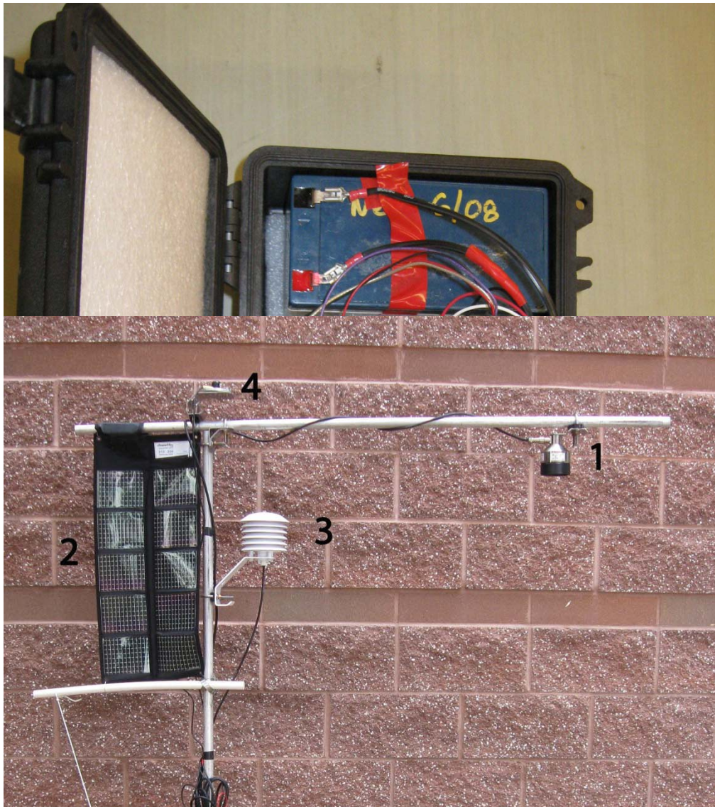
Figure 3: This is a close-up of the data-logger box. 1) Male ends of the 8 - position connectors. 2) Campbell CR200 data-logger. 3) Corresponding female end for the radiation sensor (left). 4) Corresponding female end for the sonic depth sensor (right).
