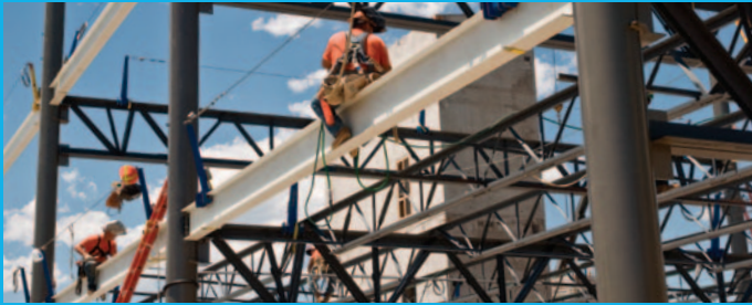
The rounded natural gas pipe will be visible in some areas of the RSF serving as a unique architectural feature. Credit: Pat Corkory/PIX 16440
