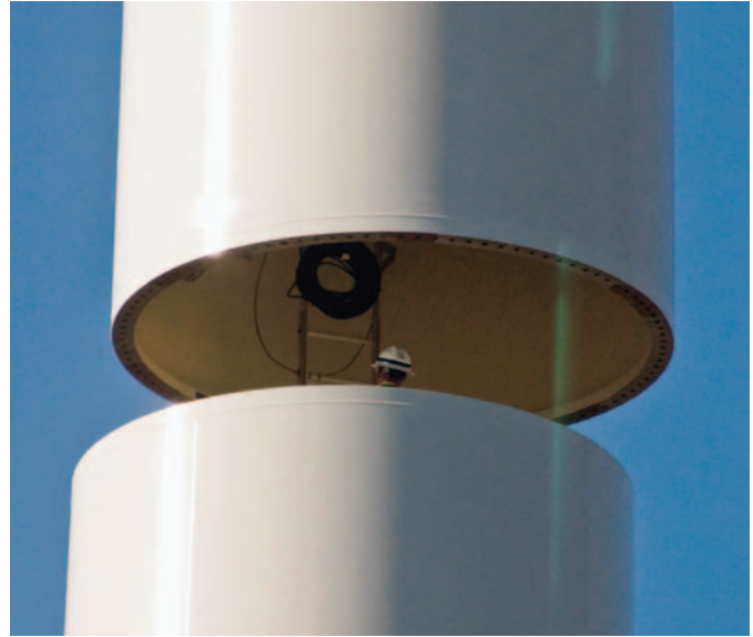
A worker waits for a crane to gently deliver a section of the metal tower supporting a General Electric 1.5 MW wind turbine at the National Wind Technology Center. Credit: Pat Corkery/PIX 16565
