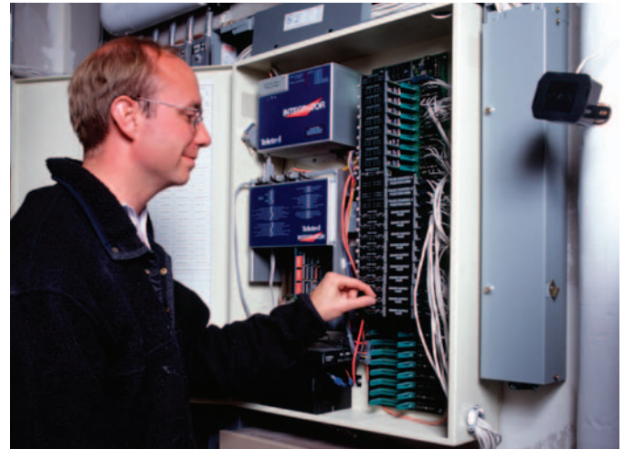
NREL Senior Engineer Paul Torcellini examines an energy management system, which helps optimize the operation of the mechanical and lighting systems in a retail store. The system controls the heating systems, ceiling fans, and lighting levels. Credit: Jim Yost/PIX 09214
