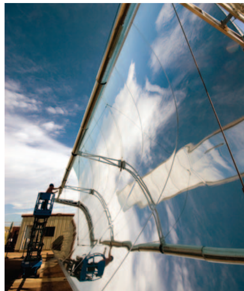
Kathleen Stynes removes the cover from the heat transfer tube on the prototype SkyTrough on South Table Mountain overlooking NREL’s Golden, Colorado, campus. Credit: Pat Corkery/Pix 16465
