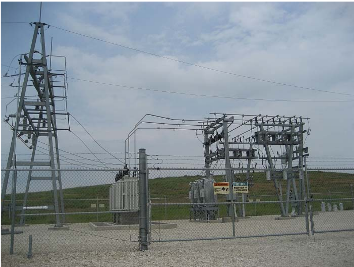
Figure 4.3-3, Looking North to Substation
