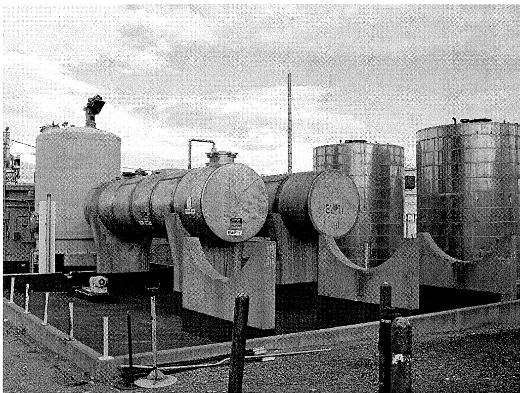
Figure 8. 311TF Tank Farm.
