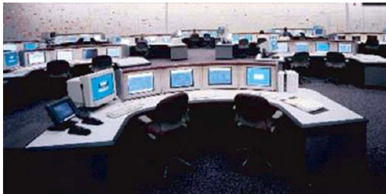
FIGURE 1.2-8 SCADA Center (Source: Argonne Staff)
