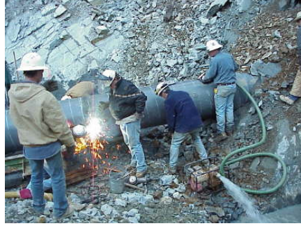
FIGURE 2.1-4 Pipeline Welding (Source: Photo courtesy of U.S. Pipeline, Inc. Reproduced with permission.)
