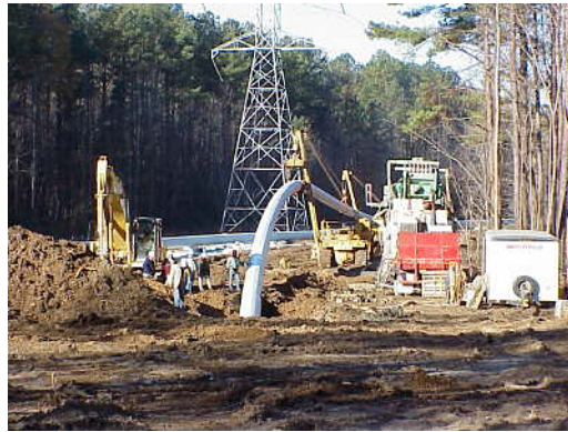
FIGURE 2.2-3 Horizontal Directional Drilling (HDD) Operation (Source: Photo courtesy of U.S. Pipeline, Inc. Reproduced with permission.)
