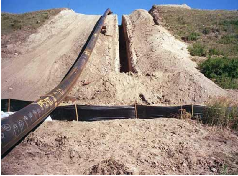
FIGURE 1.2-1 Typical Installation of a Large Transmission Natural Gas Pipe (Source: Argonne Staff)
