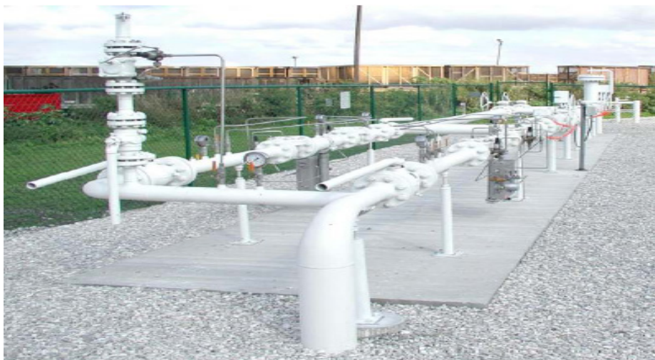
FIGURE 1.2-5 City Gate Gas Measurement and Regulation Station (Source: Argonne Staff)
