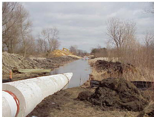
FIGURE 2.2-6 Pipeline for Wetland Installation Encased in Concrete to Counteract Positive Buoyancy (Source: Photo courtesy of U.S. Pipeline, Inc. Reproduced with permission.)
