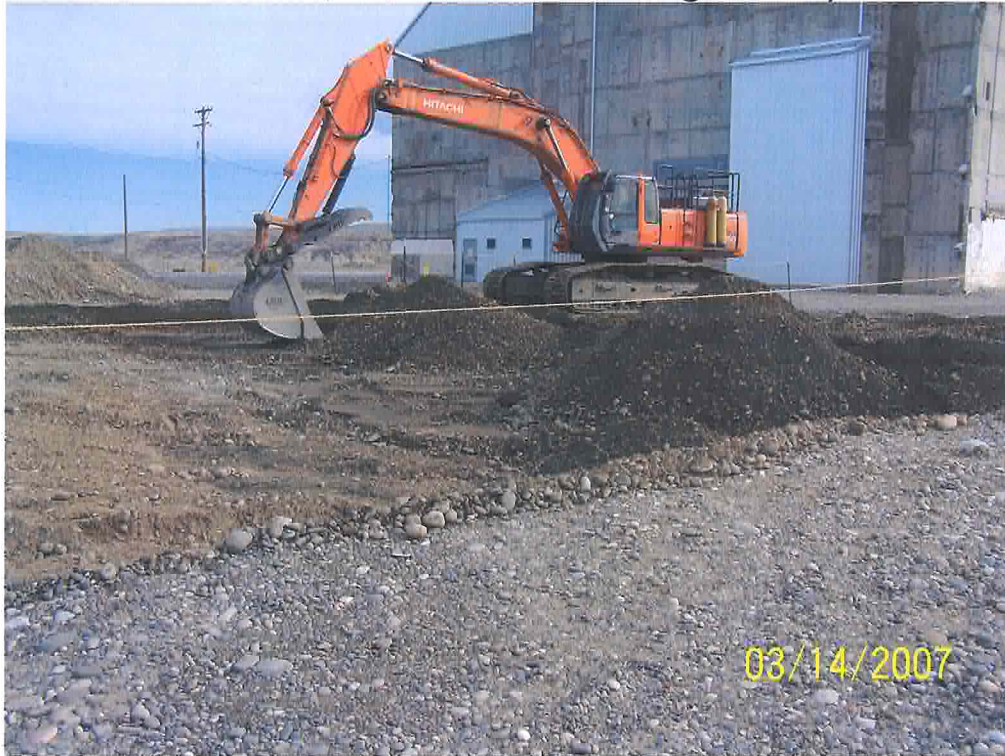
Removing overburden at 100-F-26:14 waste site. (Looking northeast; west side of 105-F Bldg. visible.)
