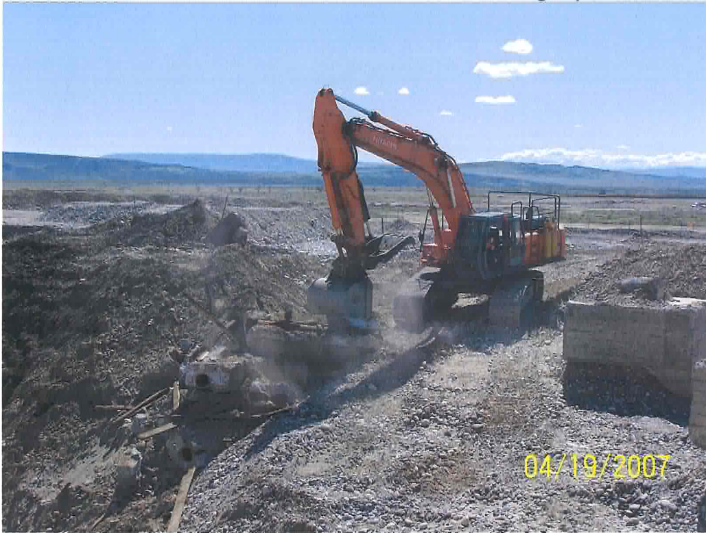
Excavation of pipe encased in concrete. (Looking southeast; former water tower foundation to the right.)
