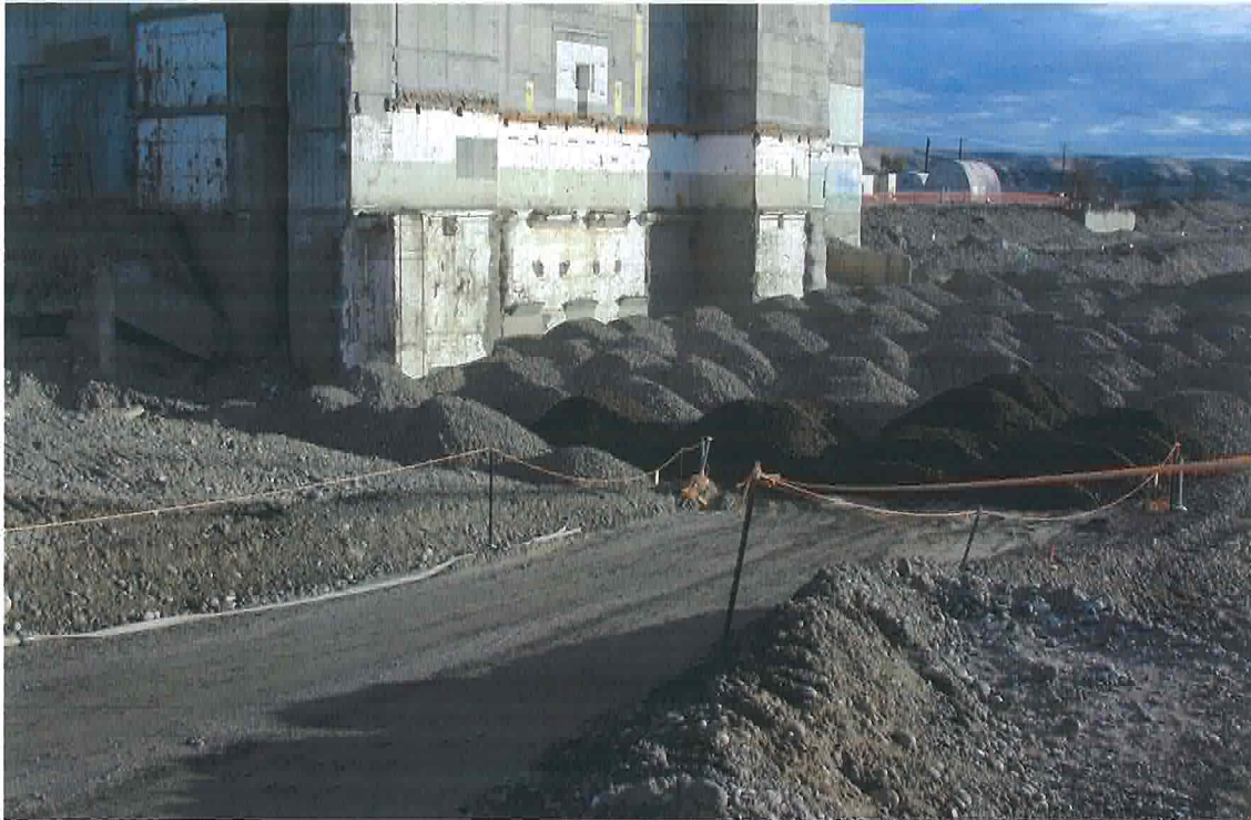
Figure 5. Ramp used for access to fuel storage basin during excavation and backfill.
