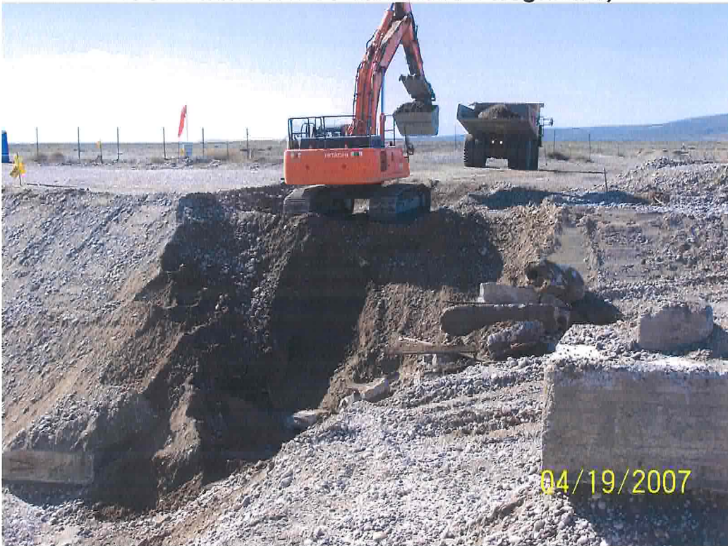
Excavating pipe encased in concrete. (Looking south; former water tower foundation in foreground.)
