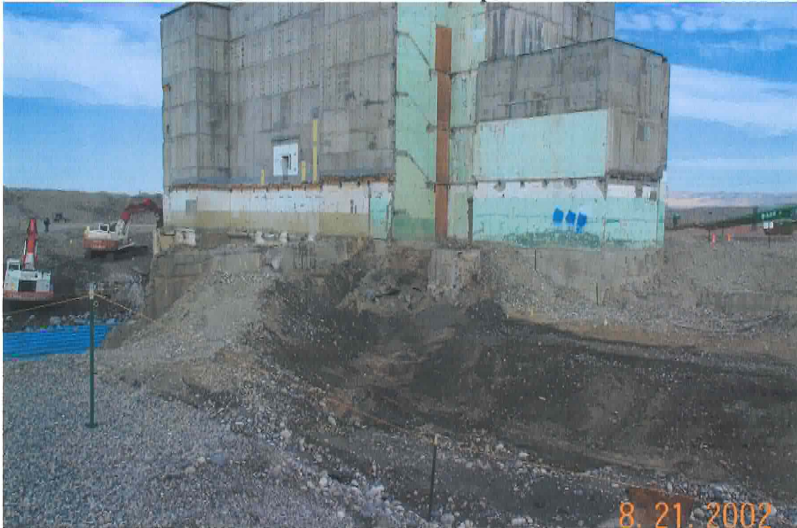
Figure 3. Excavation of Fuel Storage Basin (blue area at bottom left); excavators on ramp.
