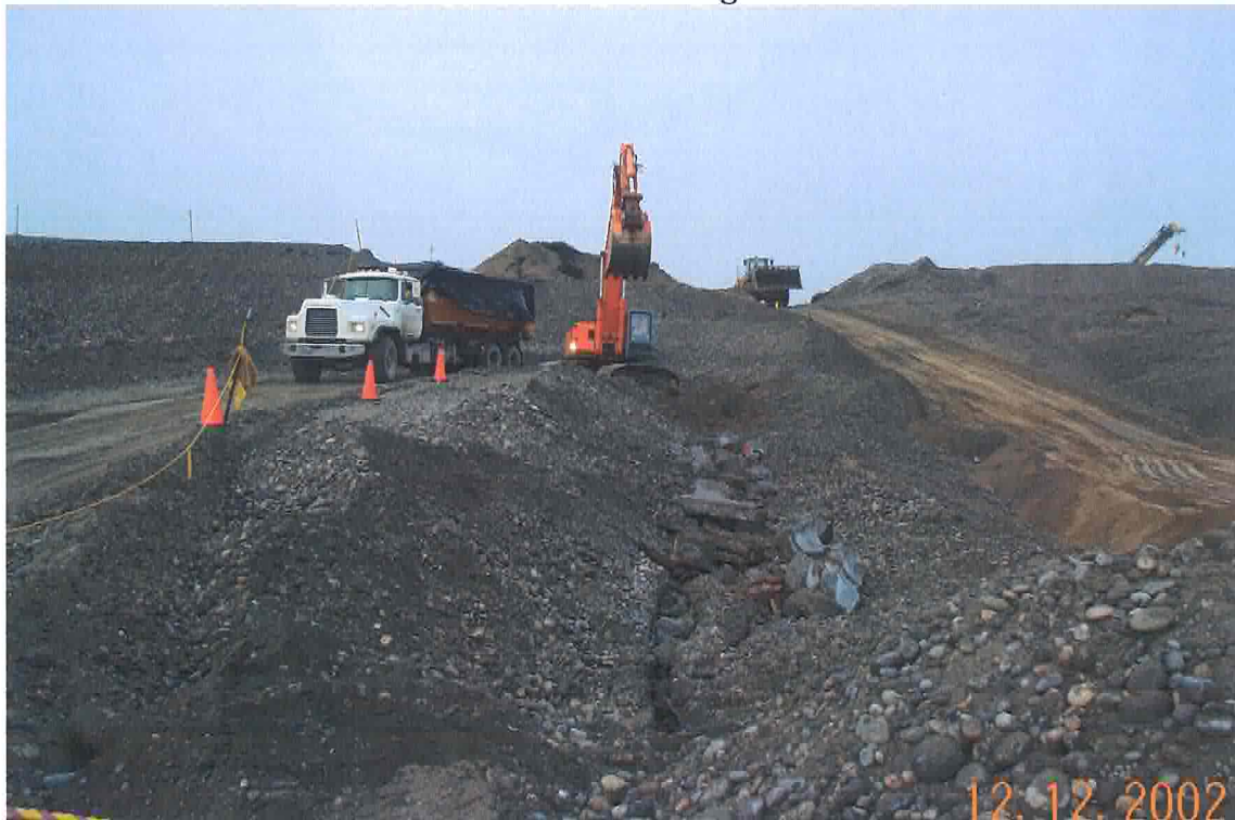
Figure 4. Excavation of 60.96-cm (24-in.) process sewer south of the fuel storage basin.
