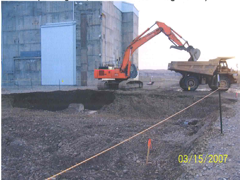
Removing overburden at 100-F-26:14/118-F-8:4 waste sites. (Looking east; west side of 105-F Bldg. visible.)
