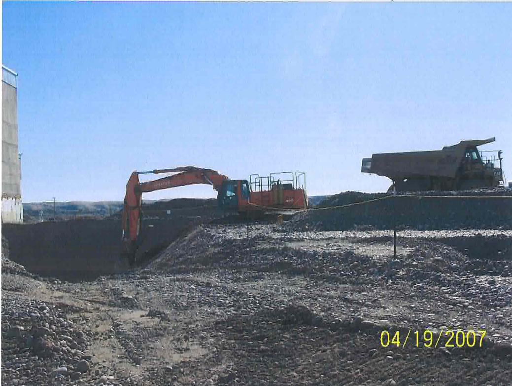
Excavating pipe encased in concrete. (Looking east; near bottom of 118-F-8:4 waste site.)
