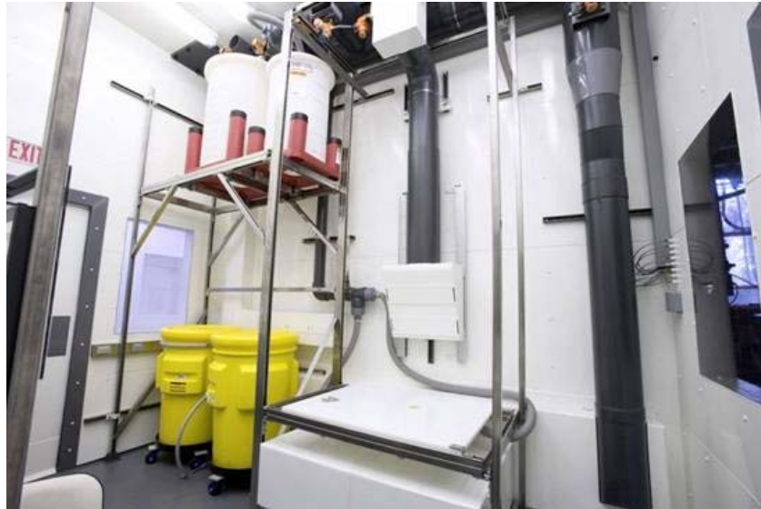
Fig. III-3. The ANL chemistry room portion of the joint ANL/FNAL SCSPF designed for electropolishing and buffered chemical polishing operations.
