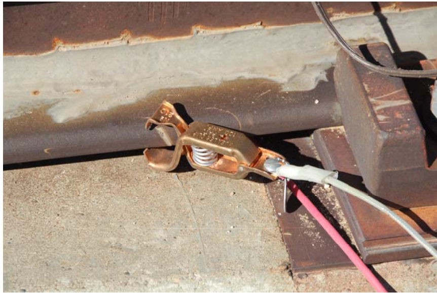
Figure 15. Ground Clamp on Sled Track Rail
