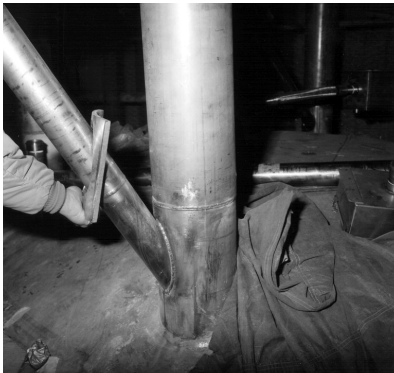
Figure A-6. Typical vessel connections on bin in the Calcined Solids Storage Facility V (81-851).
