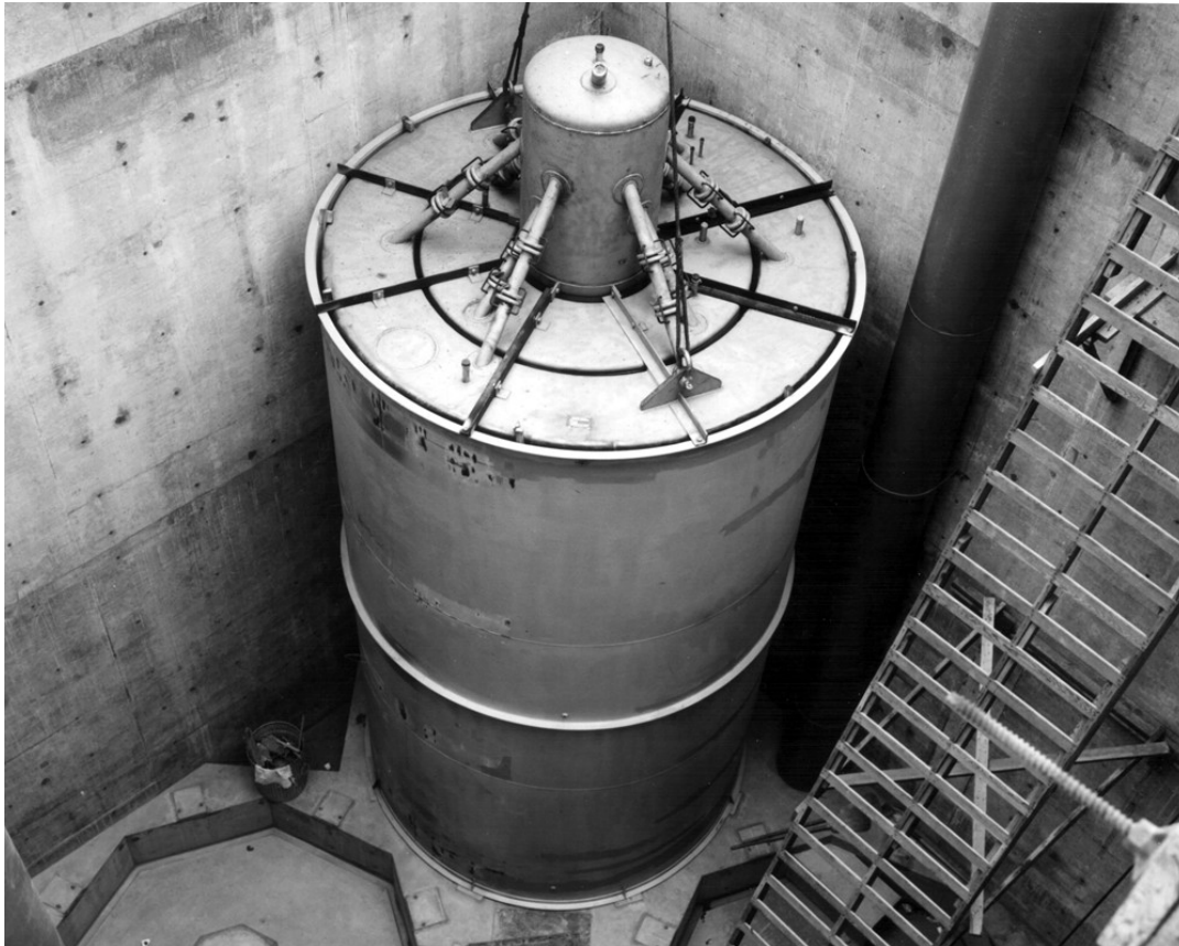
Figure A-2. Calcine storage Bin VES-WCS-115-2 in Calcined Solids Storage Facility I (59-5283).
