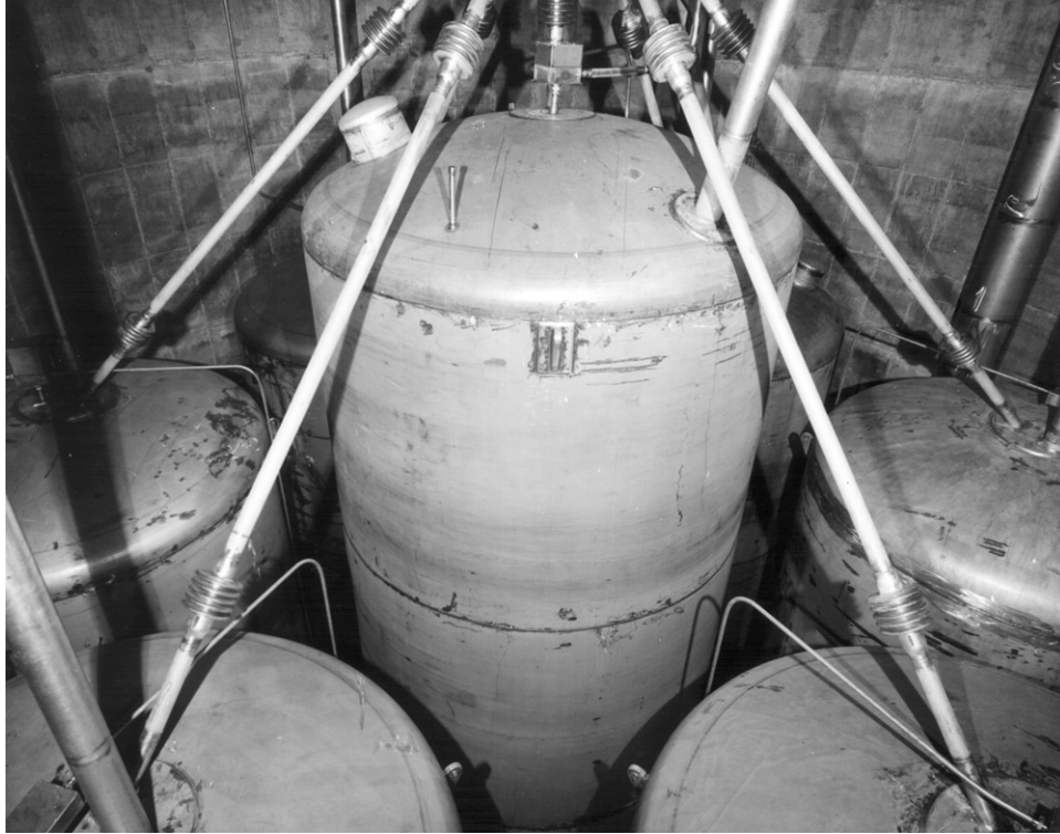
Figure A-4. Center Bin VES-WCS-139 (also known as VES-WCS-140-7) in interior of Calcined Solids Storage Facility III (71-4954).
