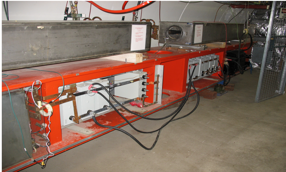
(a) Two Booster combined-function magnets on a girder
