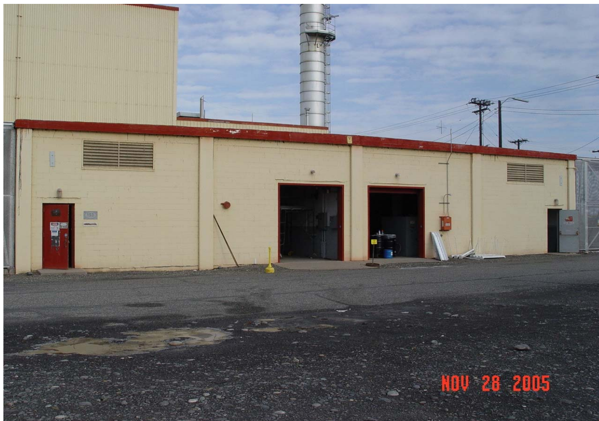
Figure 1. 153-N Electrical Substation.
