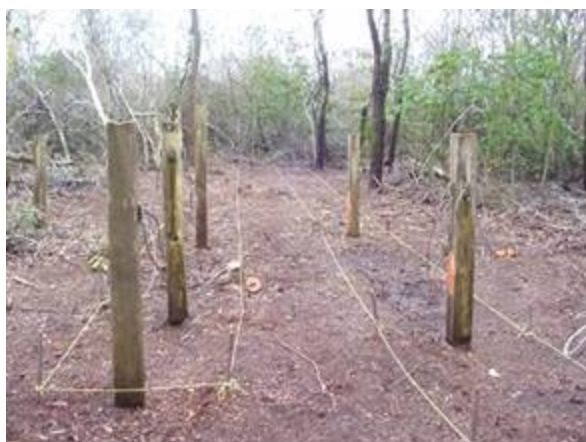
Figure 7. Looking south at 1971 trench on the left and 1970 on the right prior to excavation.
