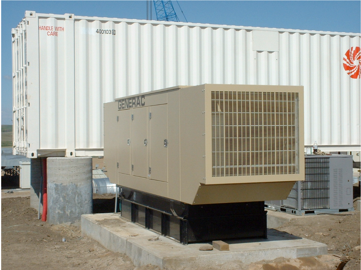
Figure 27. 225 kW Standby Generator On-Site For Emergency Backup ORMAT Modular Switchgear and Control Building in Background.
