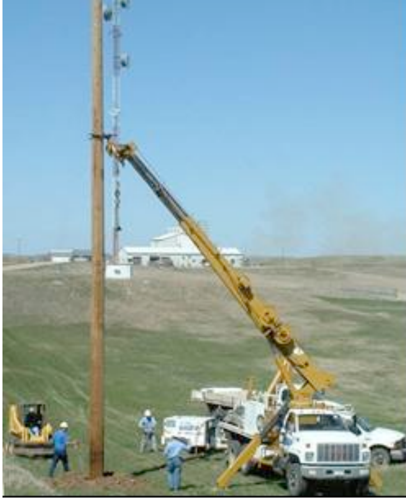
Figure 24. Feeder line from ORC to the Grid
