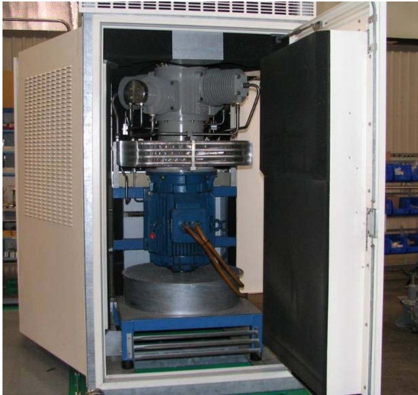
Figure 38: Oil-Free Reciprocating Compressor
