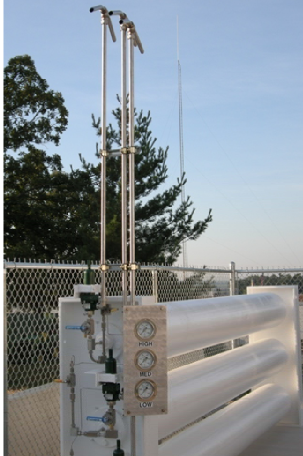
Figure 27: Traditional Three-Bank ASME Steel Vessels With Controls and Vent Line
