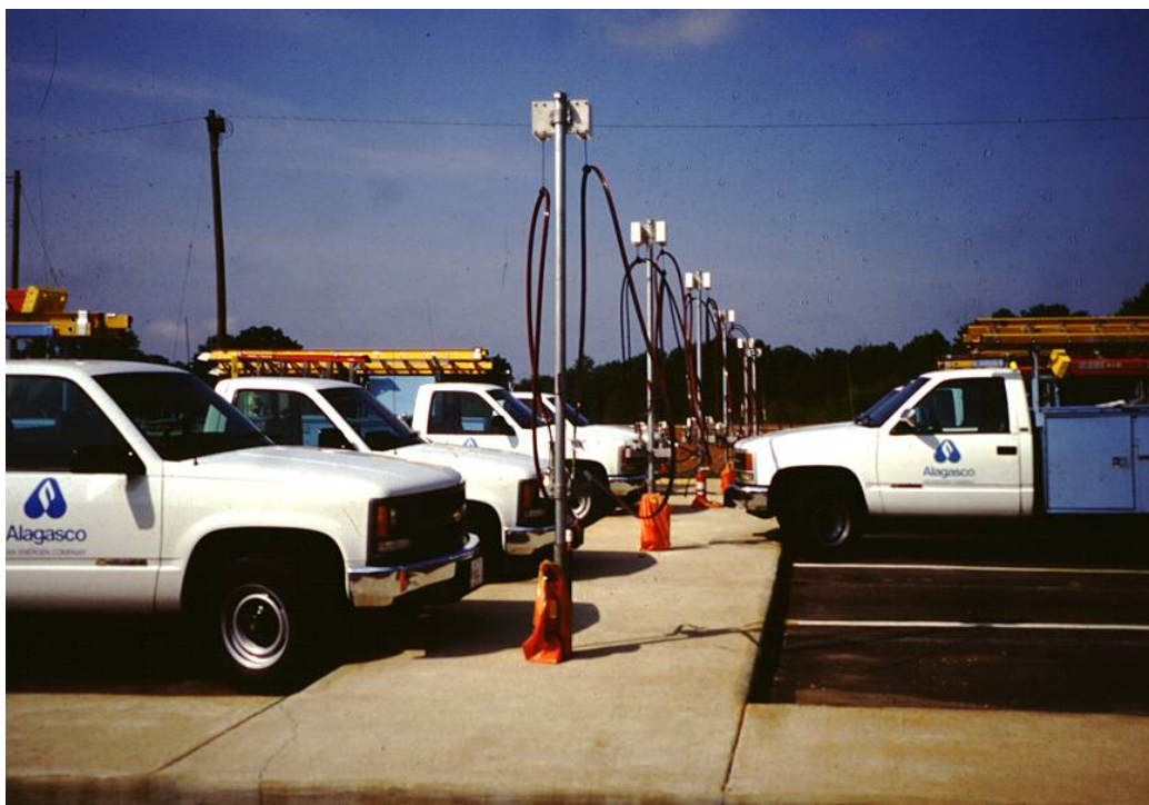
Figure 12: Time Fill Station for Centrally Fueled Fleet
