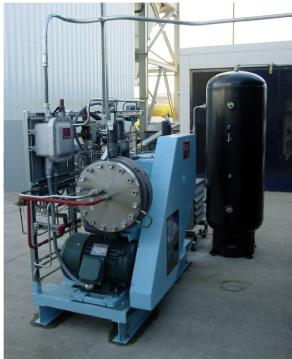
Figure 36: Two-Stage Hydrogen Diaphragm Compressor
