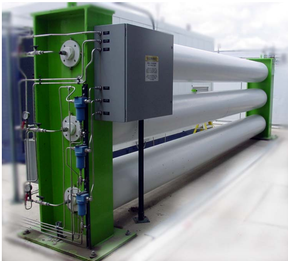
Figure 20: Three Bank Cascade With ASME Steel Pressure Vessels
