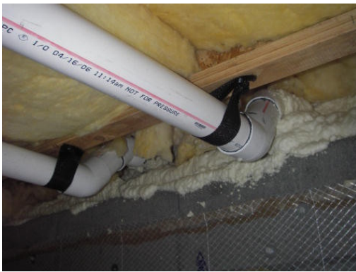
Properly Sealed Penetrations and Liner
