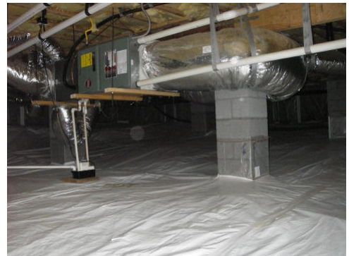
Raised HVAC System
