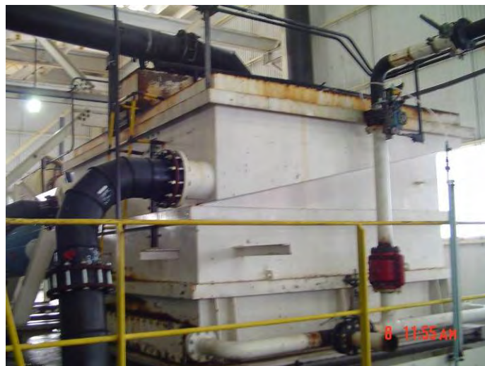
Figure 3.10. Photograph of the installed full-scale CrossFlow separator.
