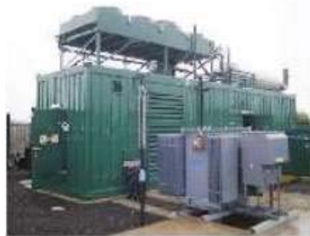
Fig. 2.4. Internal combustion generator fueled by methane gas.
