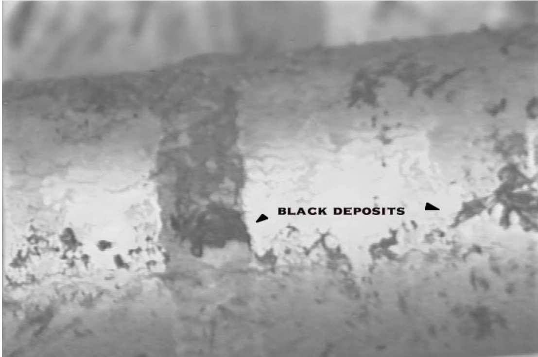
Figure D-7. Cooling coil pipe surface with deposits (PD03-0029-07). 5
