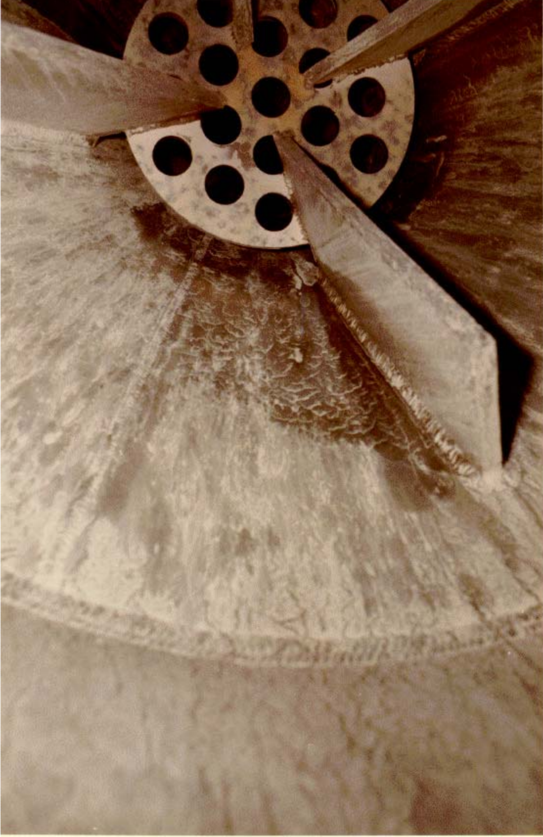
Figure A-16. Lower portion of knockout drum (VES-NCC-111) prior to decontamination. There was no calcine accumulation on the baffles or catch plate in the bottom of the vessel (81-5570).
