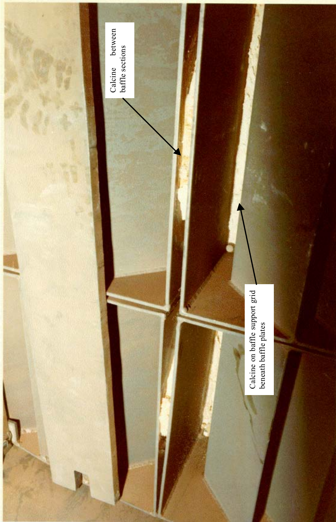
Figure B-3. Close-up view of Calciner baffle plates after decontamination showing calcine remaining between the baffle plate sections and on the baffle support grid beneath the section joints. The baffle supports were modified to eliminate the calcine residue seen in this picture (82-258).
