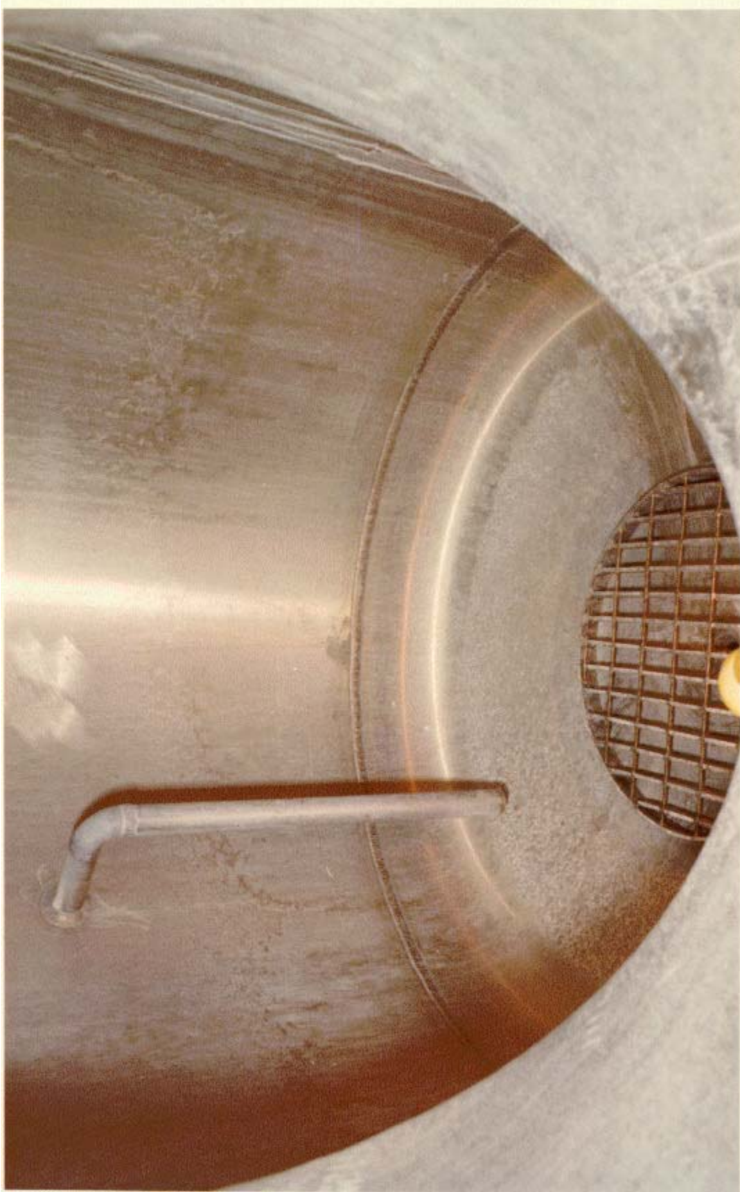
Figure A-18. View of the lower portion of mist eliminator (VES-NCC-110) before decontamination showing no calcine accumulation. The catch plate over the liquid drain line is in the lower part of the photograph (81-5568).
