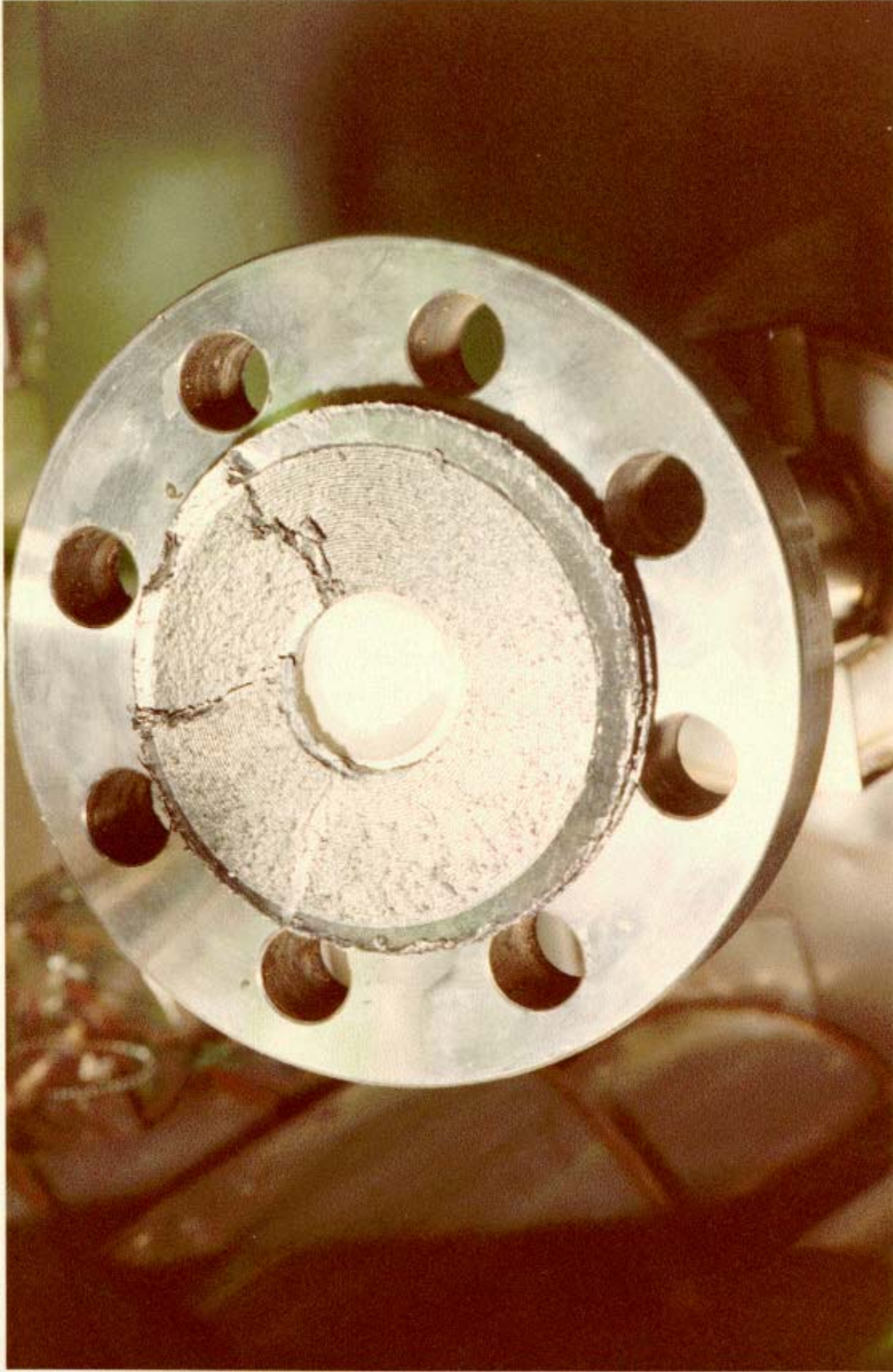
Figure A-11. The west calcine product removal line plugged with calcine prior to decontamination (81-5542).
