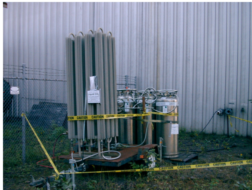
Figure 10: CO 2 tanks and evaporator at the Northshore plant. Liquid CO 2 was vaporized in the evaporator, and injected into the filter slurry as a gas
