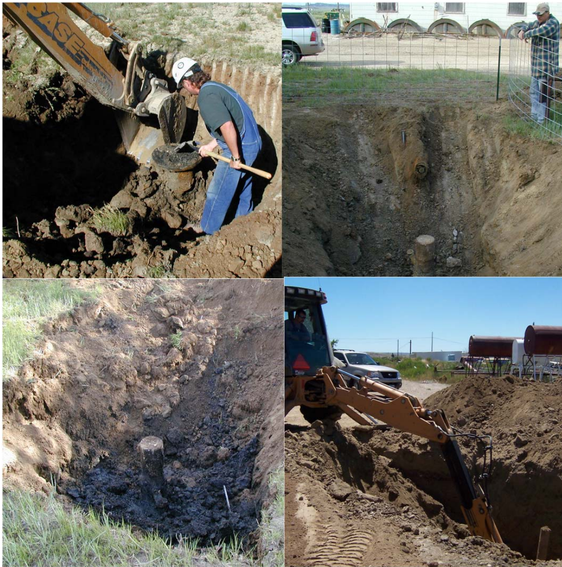
Figure 6. This collage of images shows a few examples of unmarked abandoned wells that were located using GIS and magnetometry then verified by excavation in Midwest, Wyoming.
