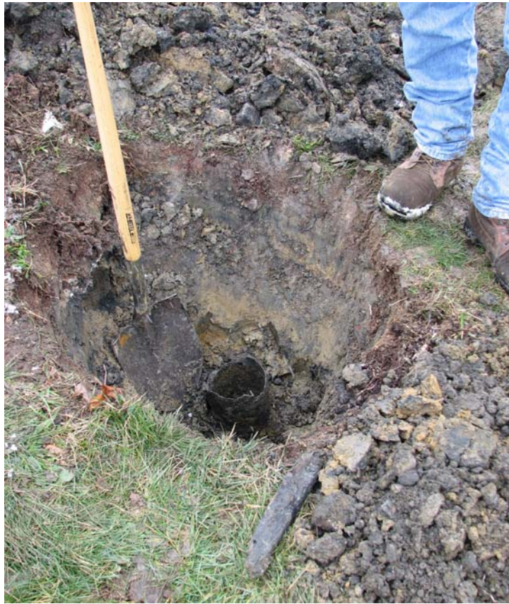
Figure 11. UAW excavated in Versailles Borough, PA. This well was first detected by methane measurements and subsequently by magnetometry
