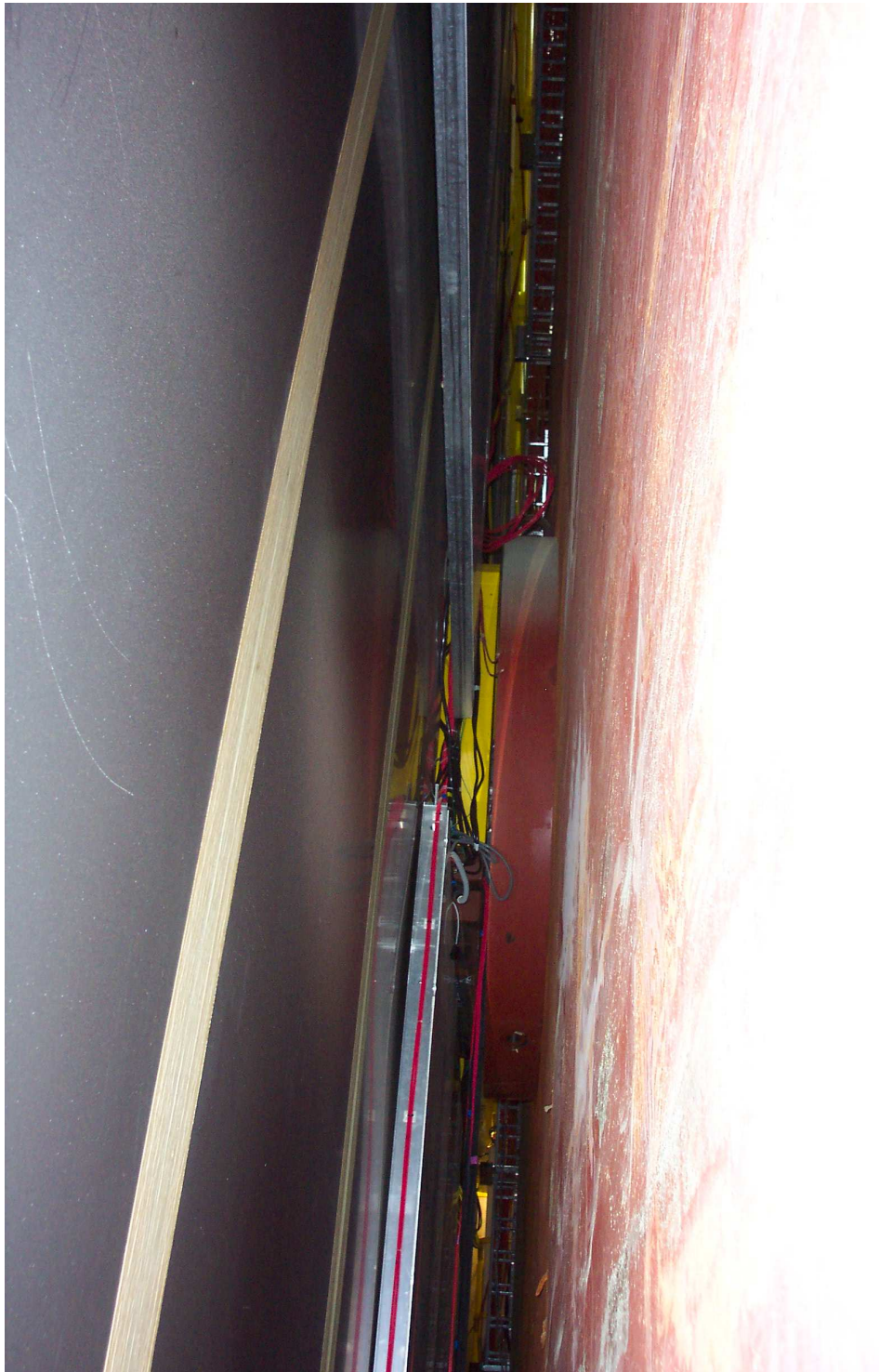
Figure 3.63: Picture of the available space for the installation of RPC2N between the muon magnet(right) and the muon wall(left). The muon magnet donut is visible in the center of the picture.
