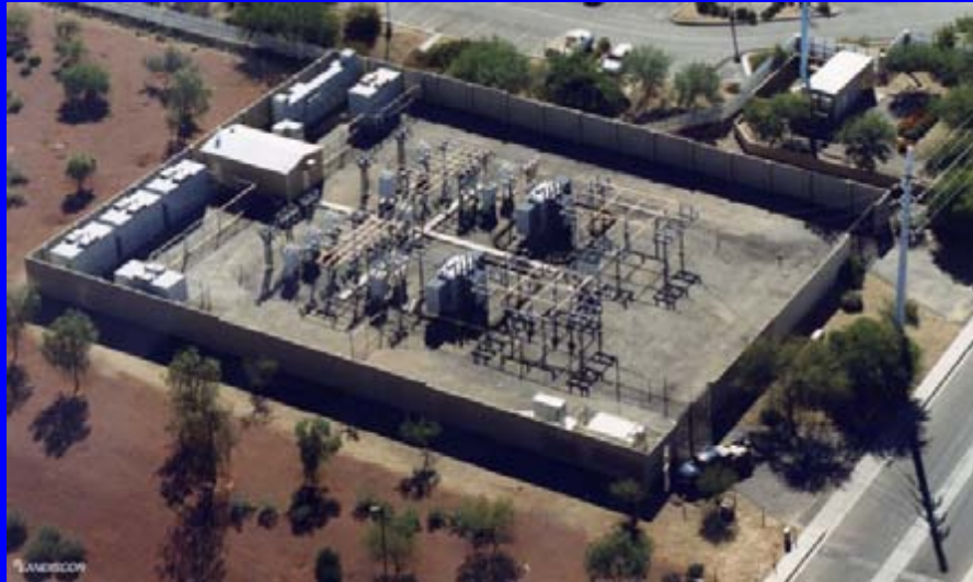
10 MW - 30 sec System at AZ Microchip Plant
