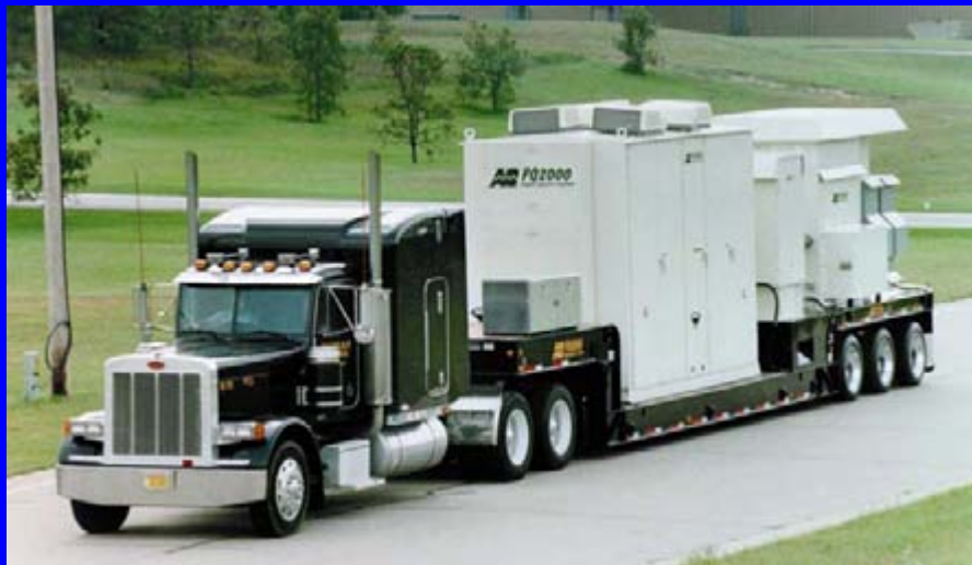
2 MW – 15 sec Mobile Battery System
