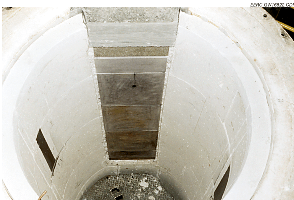
Exhibit 11-57 Photograph of New Monofrax M tiles Installed on the RAH Panel in January 1999
