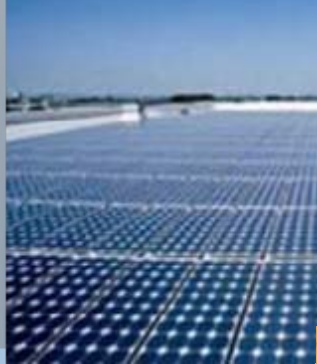
PowerLight PowerGuard® Rooftop 536 kW, Toyota Motor Corp.,
