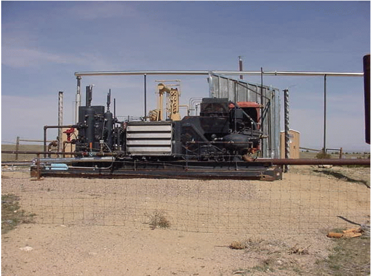
Figure 4. Natural Gas Fueled Compressor C2, Burnt Wagon Field
