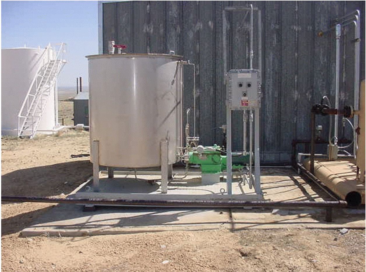
Figure 6. Methanol Injection Unit, Burnt Wagon Field
