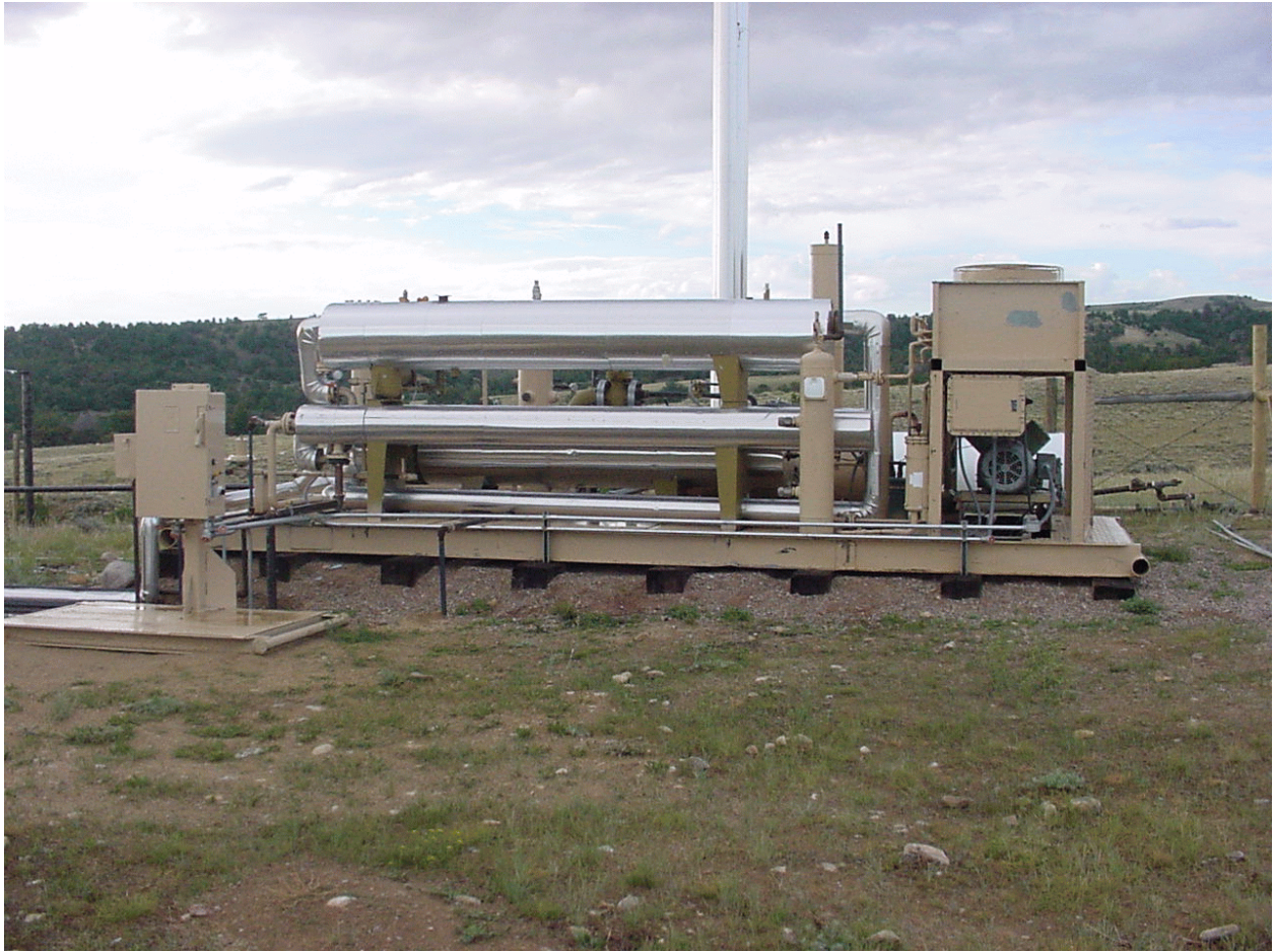
Figure 5. Cryogenic Gas Processing Unit, Burnt Wagon Field
