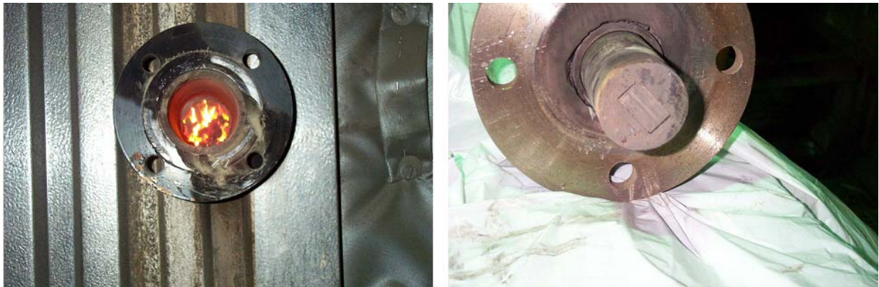
Figure 11. Probe port 2 after removal of the EN sensor (left) and appearance of the sensor elements (right).
