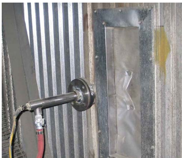
Figure 5. Corrosion sensor installed at location 2 on the south wall.
