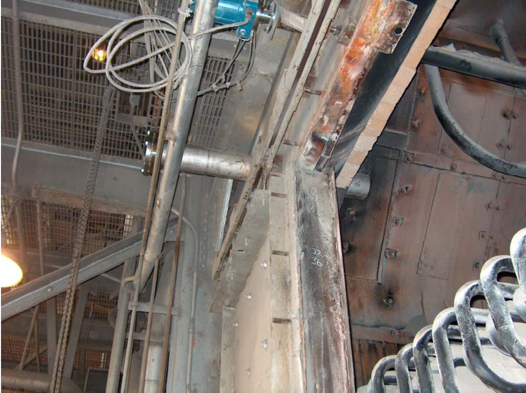
Figure 42. Inlet port installed at economizer exit at Plant Gadsden.
