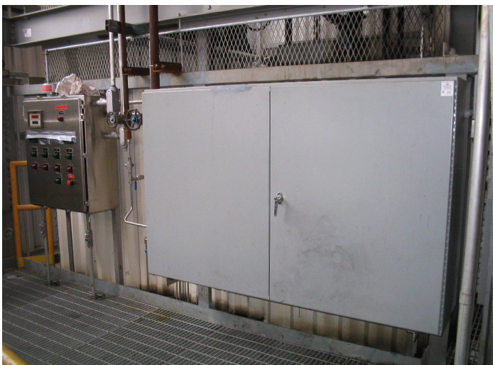
Figure 1a. Equipment Shipped to Test Site – Control Boxes
