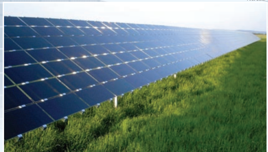
First Solar CdTe thin-film modules in a 1.3-MW solar field, Germany.
