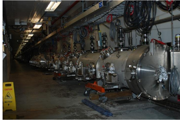
Figure 4: C100 cryomodule in the Tunnel
