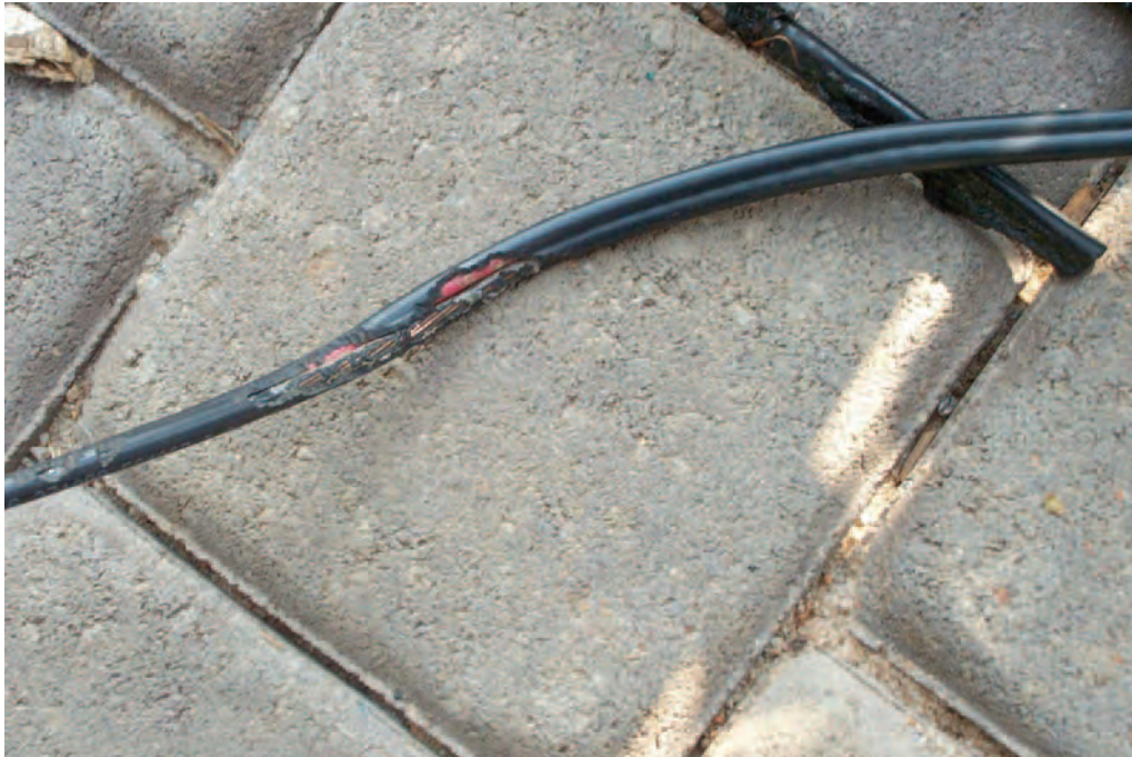
Photo #3 Chewing damage to an AC wiring cable of a PV system (J. Wiles)
