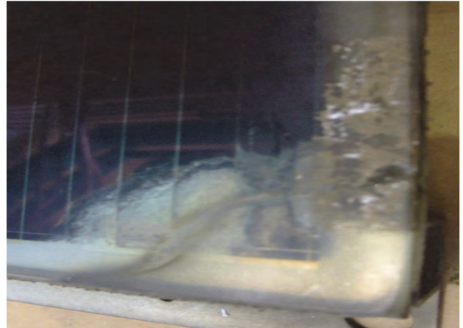
Broken Glass Leading to Corrosion
