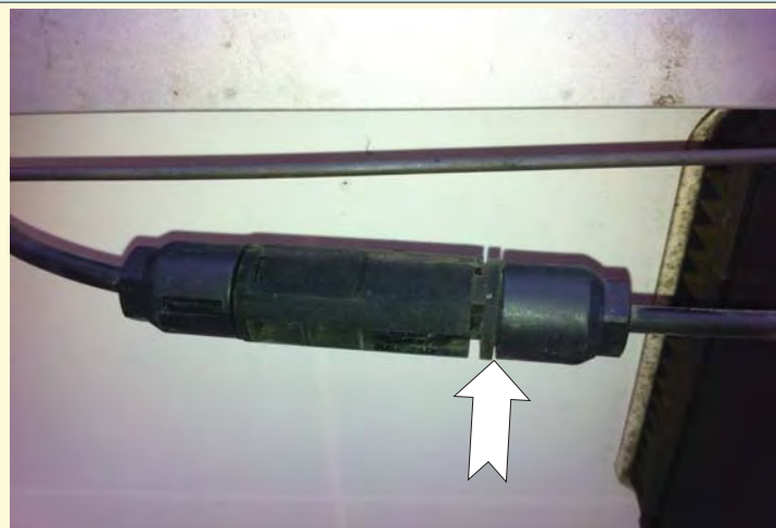
3. Gap of 2-3 mm opens up between mating connectors without any obvious external damage, external stress or fracture in latches
