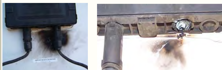
2. Connector failures at junction box
