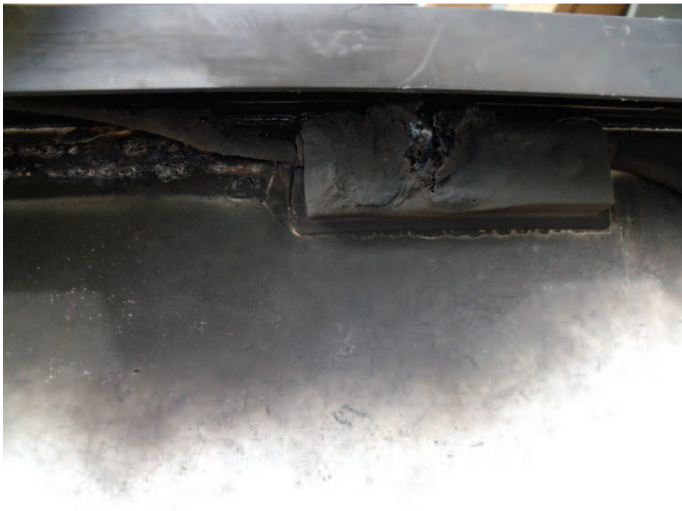
Photo #6 After fire caused by squirrel family gnawing on dc conductors (N. Soleil)
