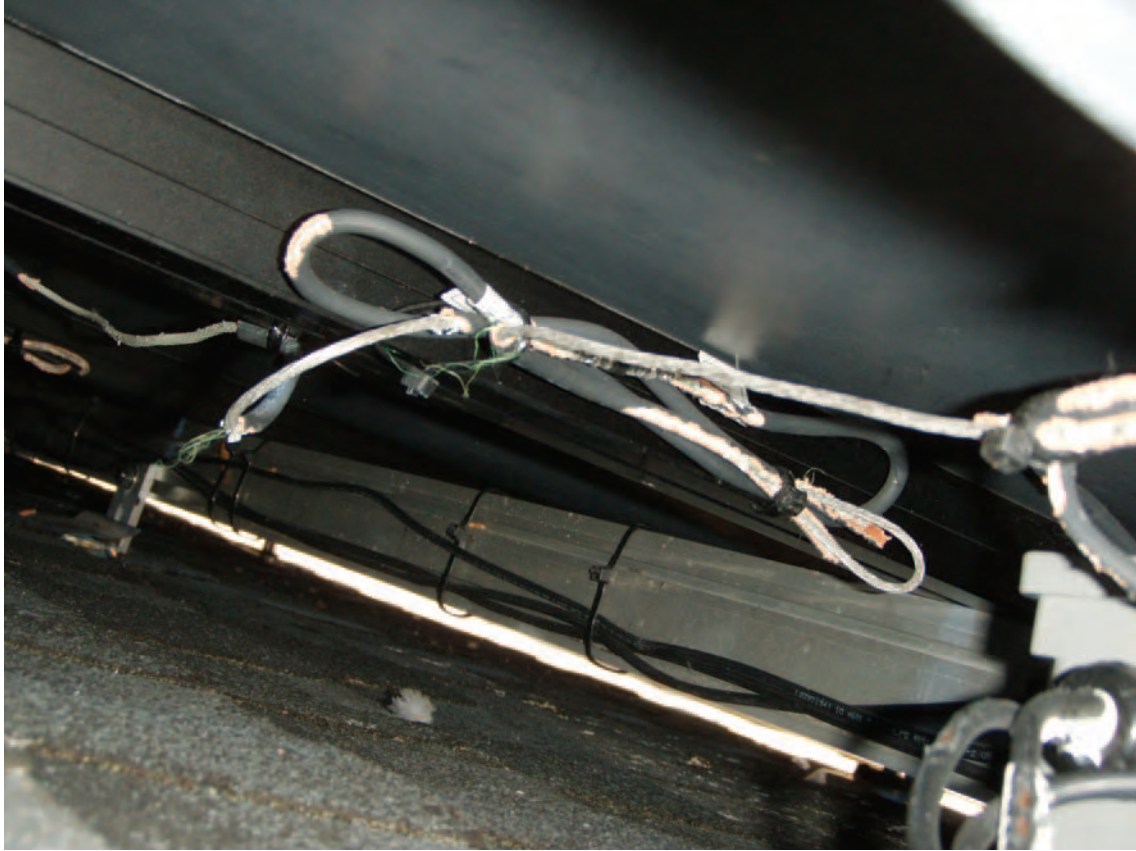
Photo #1 DC wires damaged by rodents (J. Wiles)
