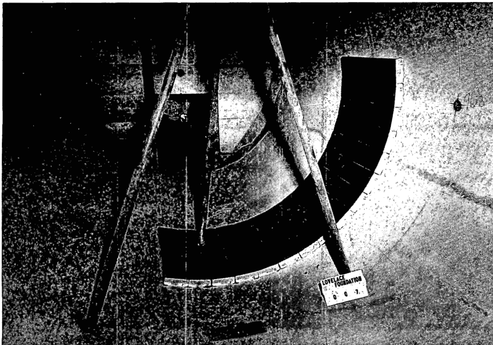
Fig. 4.159— Typical installation of missile absorber in conduit type shelters. See Ref. 4 for details of shelter construction.
