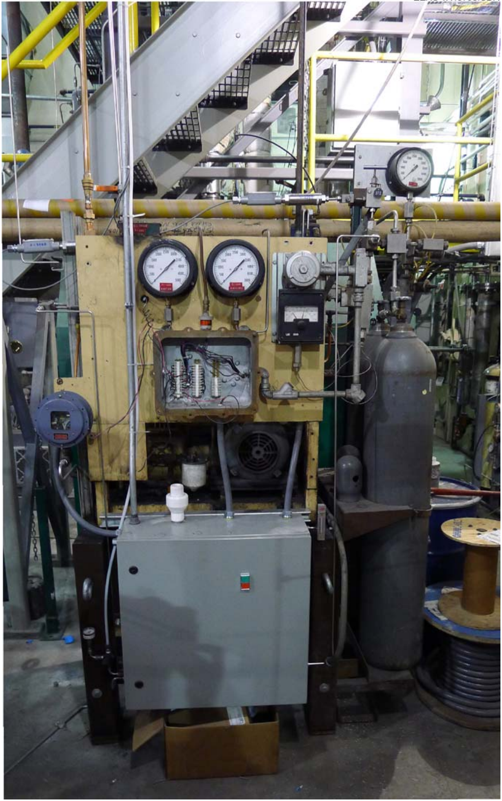
Figure II-8. MCL Pilot Plant Nitrogen Compressor System.
