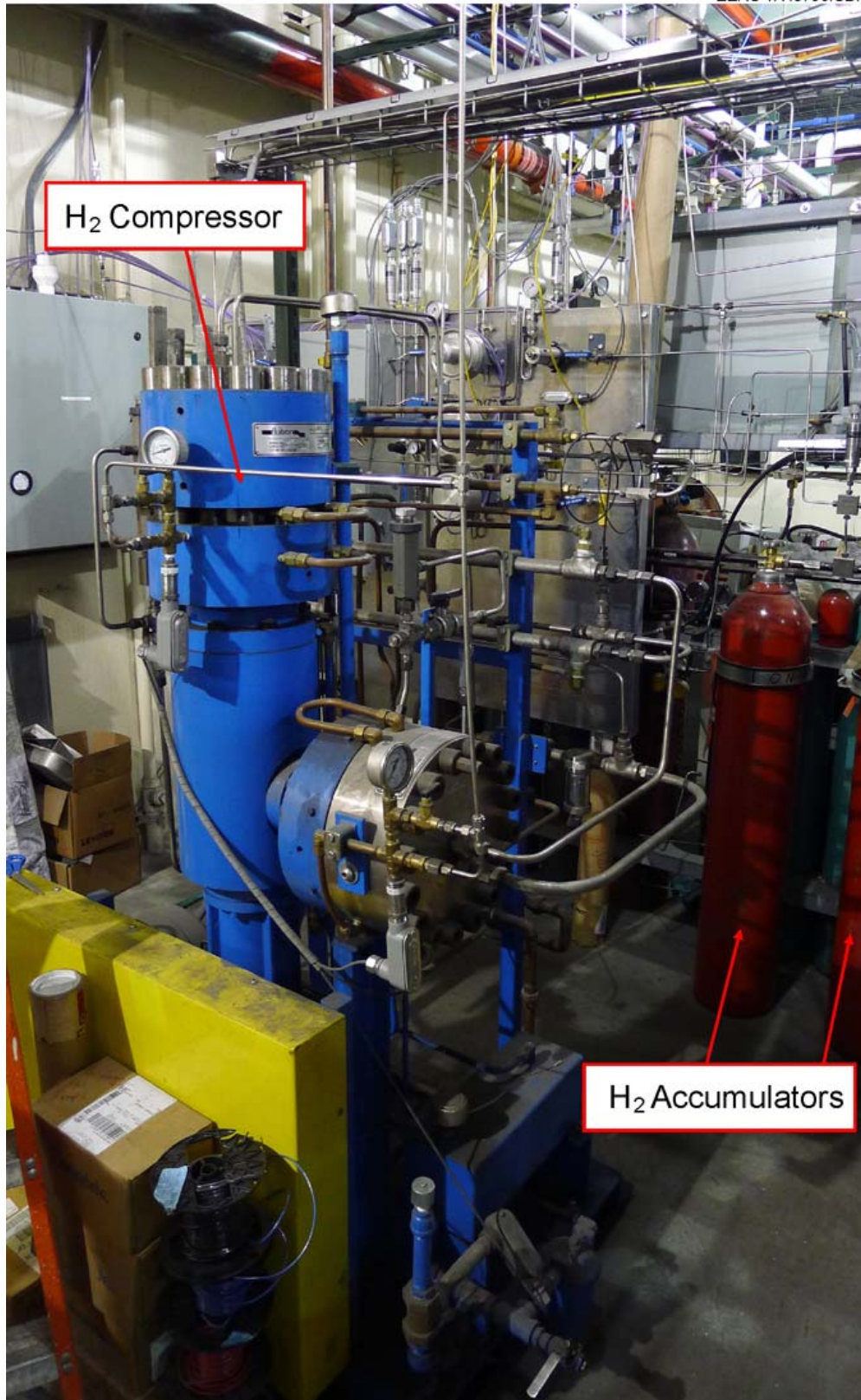
Figure II-7. MCL Pilot Plant Hydrogen Compressor System.
