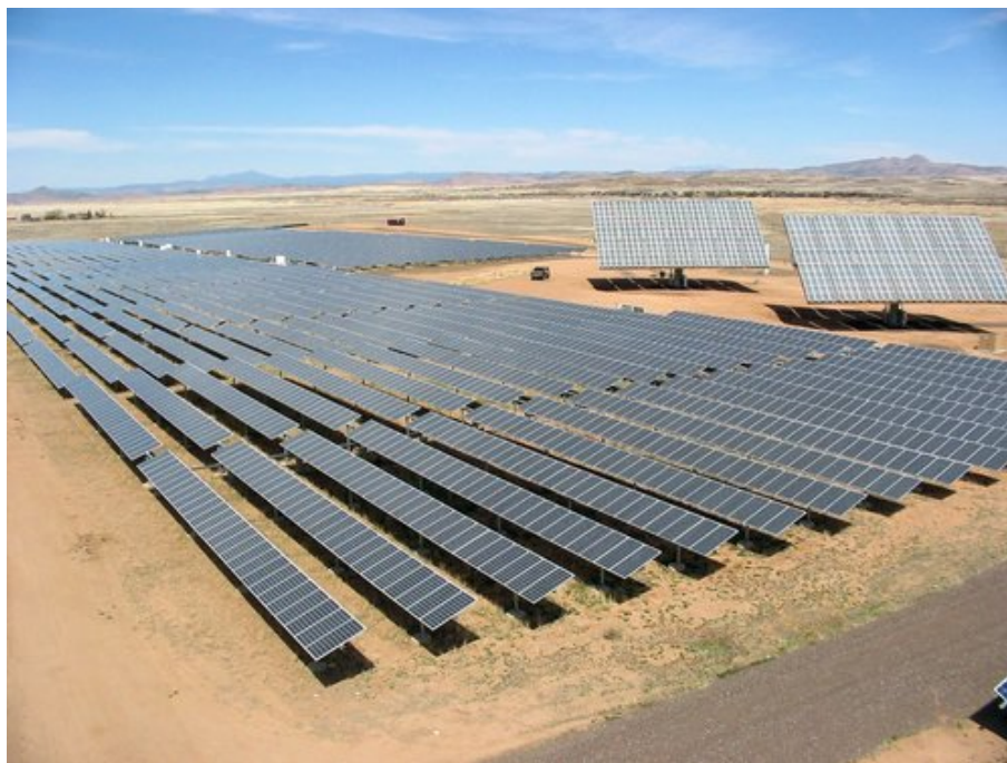
Figure 3-33 Utility-Scale PV, Single-Axis Tracking Collector Totaling 2 MW at Prescott, Arizona (Source: NREL 2012e)
