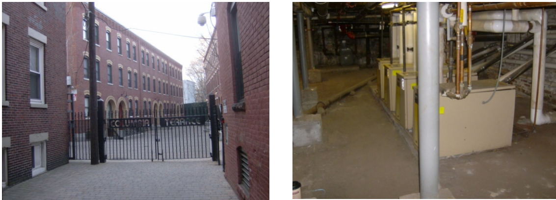
Figure 1. Exterior view of Building 4 and typical basement boiler room
