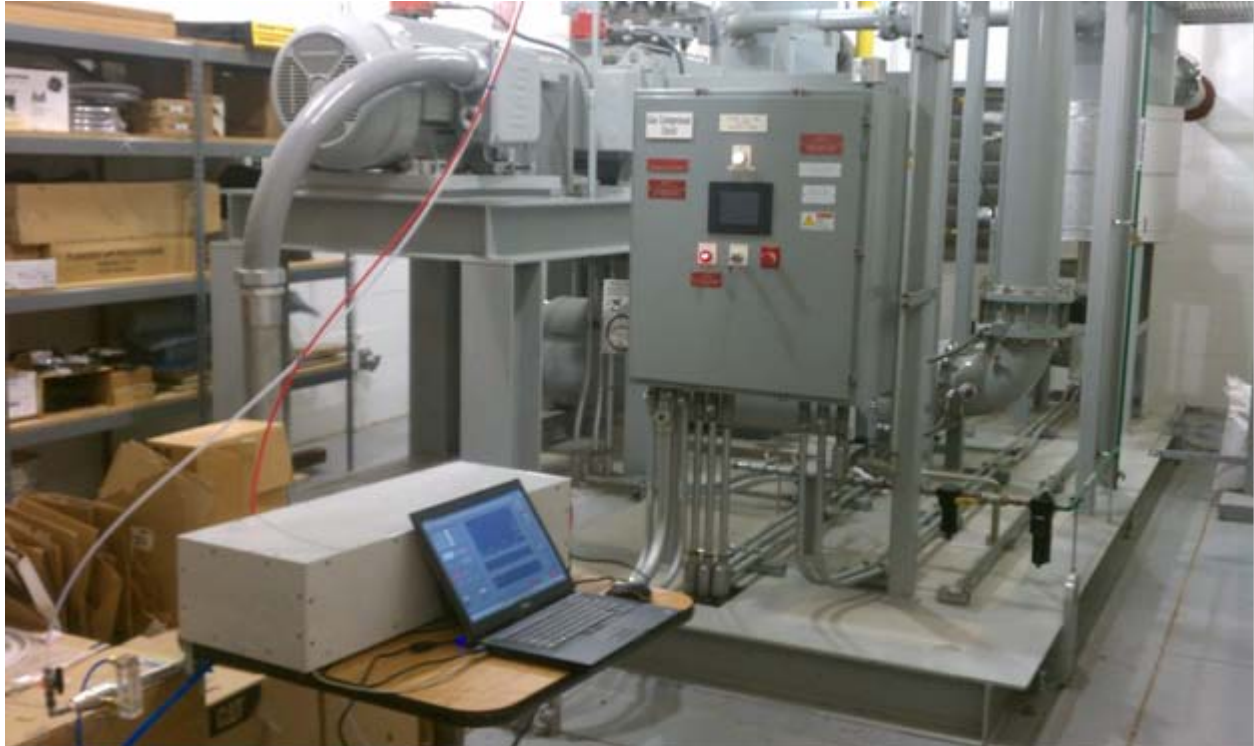
Figure 44. GQS setup at Bath Landfill, Steuben County, New York,
