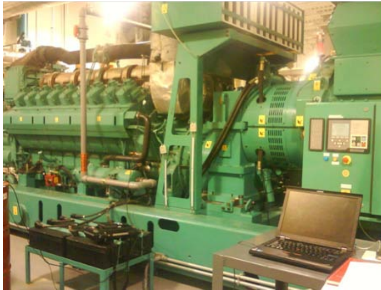
Figure 43. A lean burn, low BTU, internal combustion reciprocating stationary engine at the Bath Landfill, Steuben County, New York. As typically, this lean-burn engine is also turbocharged and aftercooled. This is a V18, 91 L engine producing 2 MW power and can run safely on landfill gas containing as low as 40% methane (~ 400 BTU/SCF).
