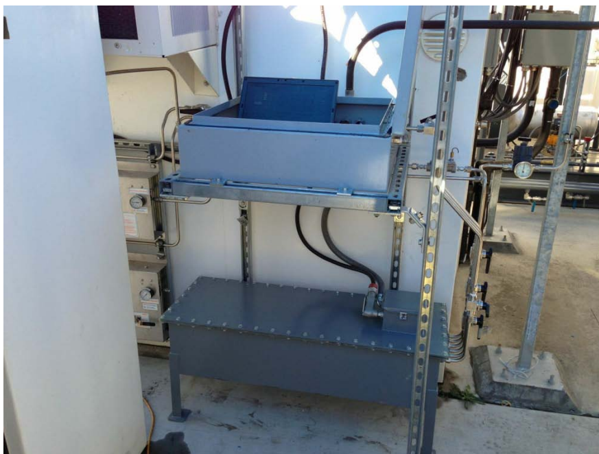
Figure 5 Photograph of GQS Setup at Escondido WWTF
