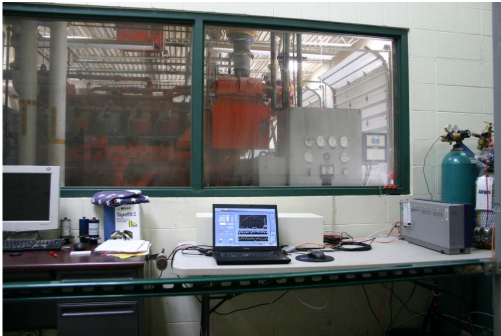
Figure 37. Photograph of the GQS installation at Glacier Ridge
