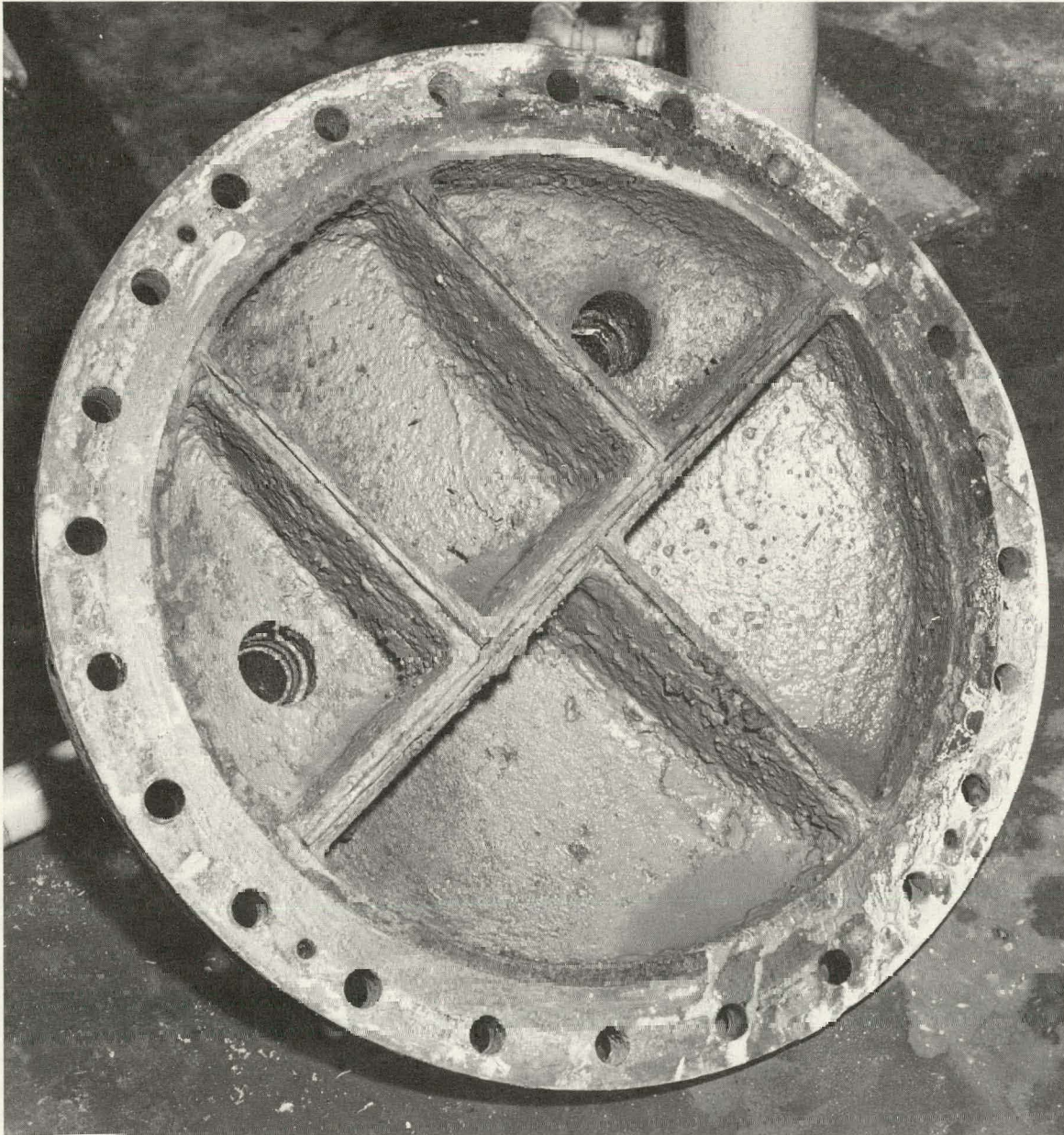
Figure 6. HEAD OF THE PLANT AIR COMPRESSOR.
