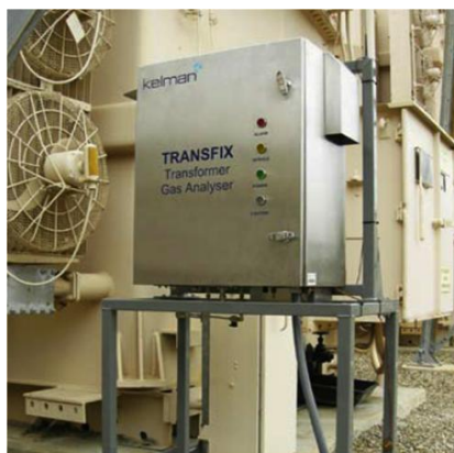
Figure 11. Kelman Transformer Gas Analyser installed on Harris transformer.
