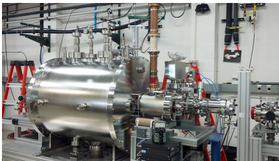
Figure 1: Electron gun installed in vault.
