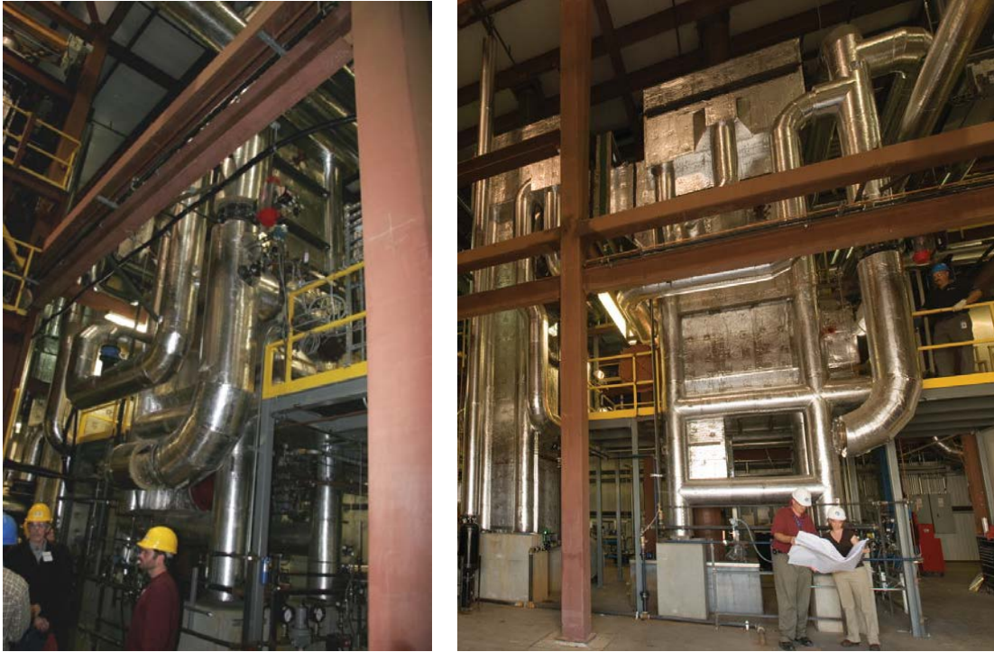
Figure 116. B&W Boiler simulator
