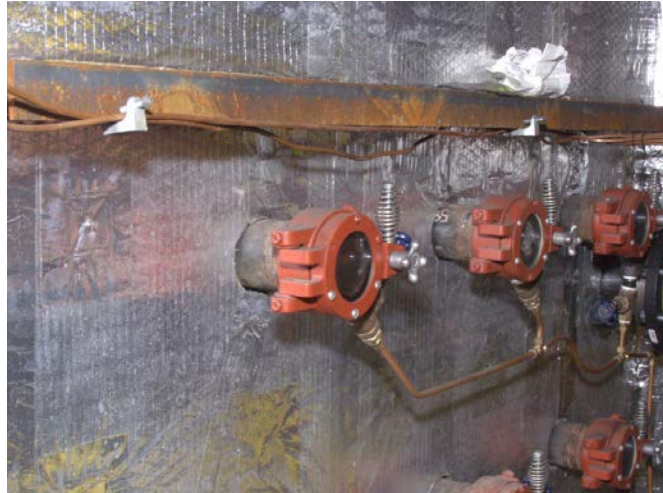
Figure 118. Access to chamber through viewports
