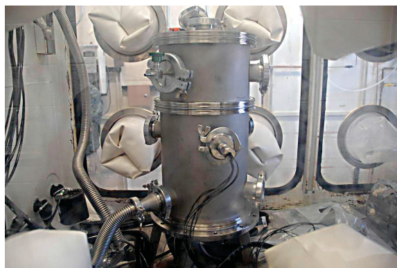
Figure 29. Glovebox Advanced Casting System installed and assembled in the Casting Laboratory glovebox.
