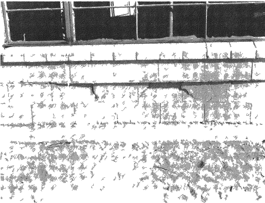
Fig. 3.20 — Damage under front window of one-story reinforced lightweight concrete-block house (31.1-f1) at 4700 ft, postshot.
