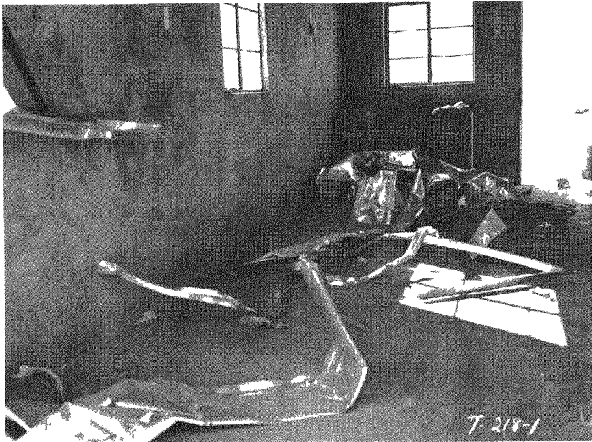
Fig. 3.16—Fragments of the garage door on the precast lightweight concrete house (31.1-e1) at 4700 ft, postshot.
