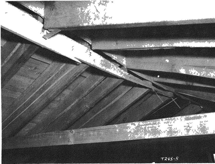
Fig. 3.41 —Failure of the ridge board in the roof framing in the two-story frame (strengthened) house (31.1-b2) at 7800 ft, postshot.
