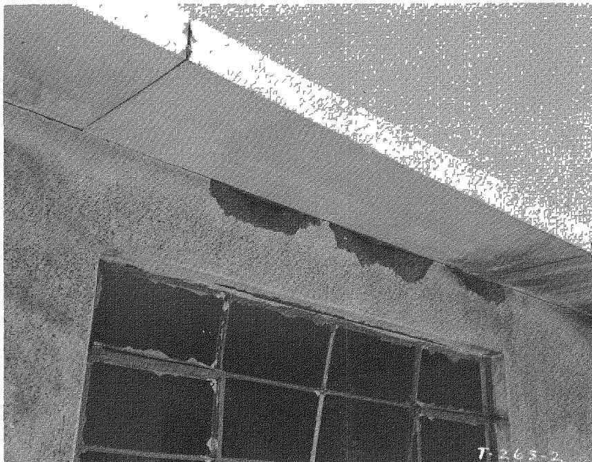
Fig. 3.12 —One-story precast lightweight concrete house (31.1-e1), postshot, showing the spalling of the concrete on the front wall at the steel lug attachments due to lifting of the roof slab by the blast.
