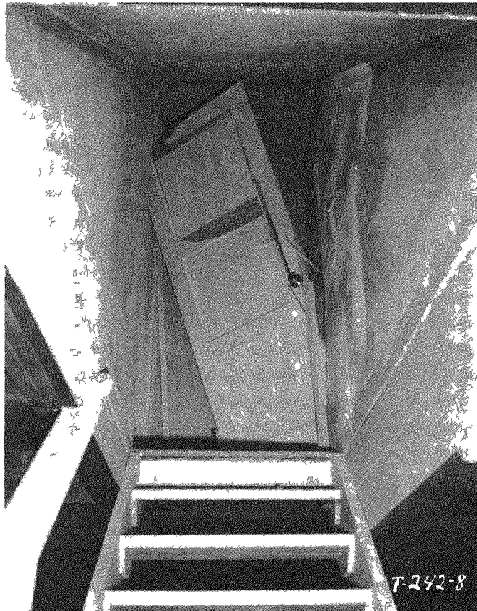
Fig. 3.29—Two-story frame house (31.1-b1) at 5500 ft, postshot, showing first-floor stair door to basement blown through plywood wall covering.
