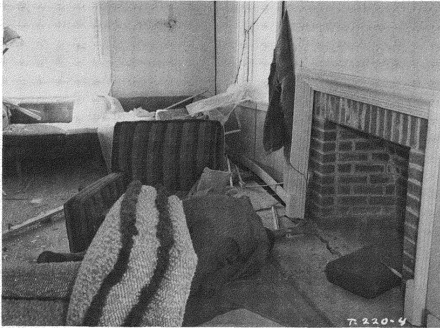
Fig. 3.25—Looking toward rear of living room in the two-story frame house (31.1-b1) at 5500 ft, postshot. The exterior wall to rear of chimney bulged several inches and pulled away from floor framing. Note split hearth.
