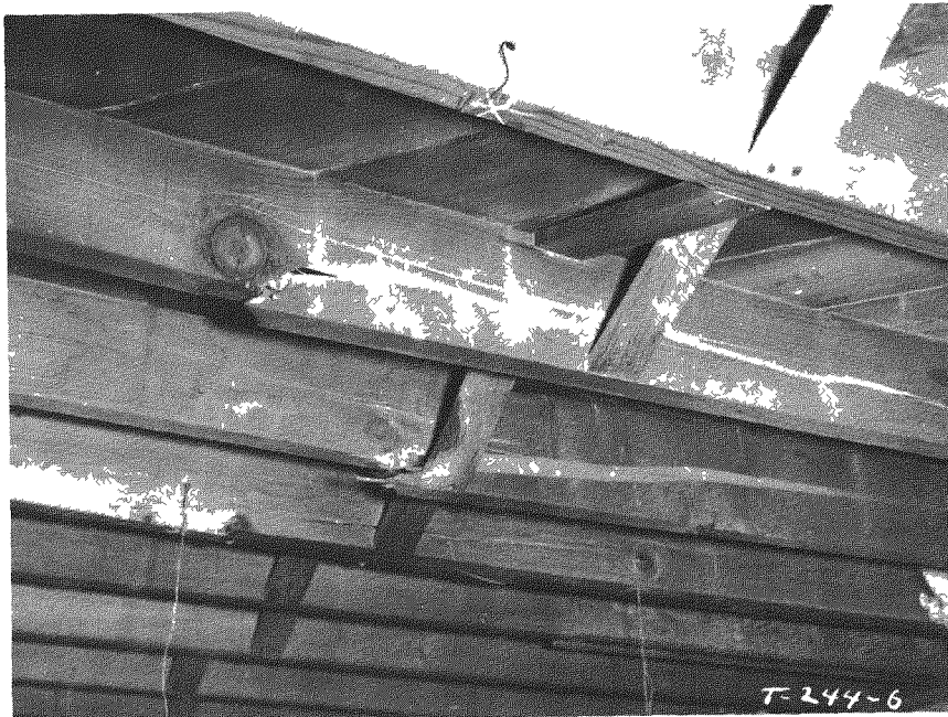
Fig. 3.44 — Fractured first-floor joists under living room in two-story brick house (31.1-a2) at 10,500 ft, postshot.
