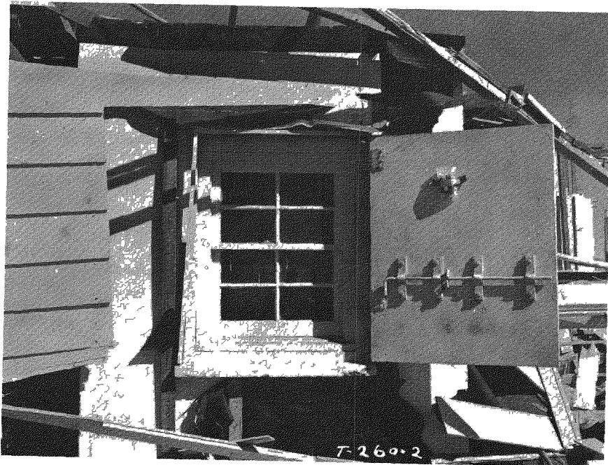
Fig. 3.8—One-story frame rambler house (31.1-c1) at 4700 ft, postshot, showing the blast shutter opened and the window of the bathroom shelter.
