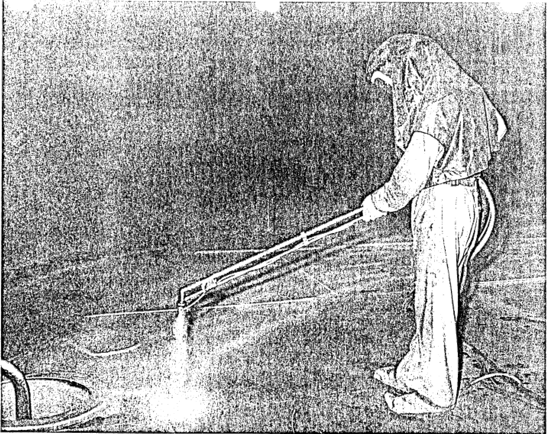
FIGURE 4-3. Application of Glassflake GF-202 to Tank Floor Using Pole Gun. (Glassflake Inter-
