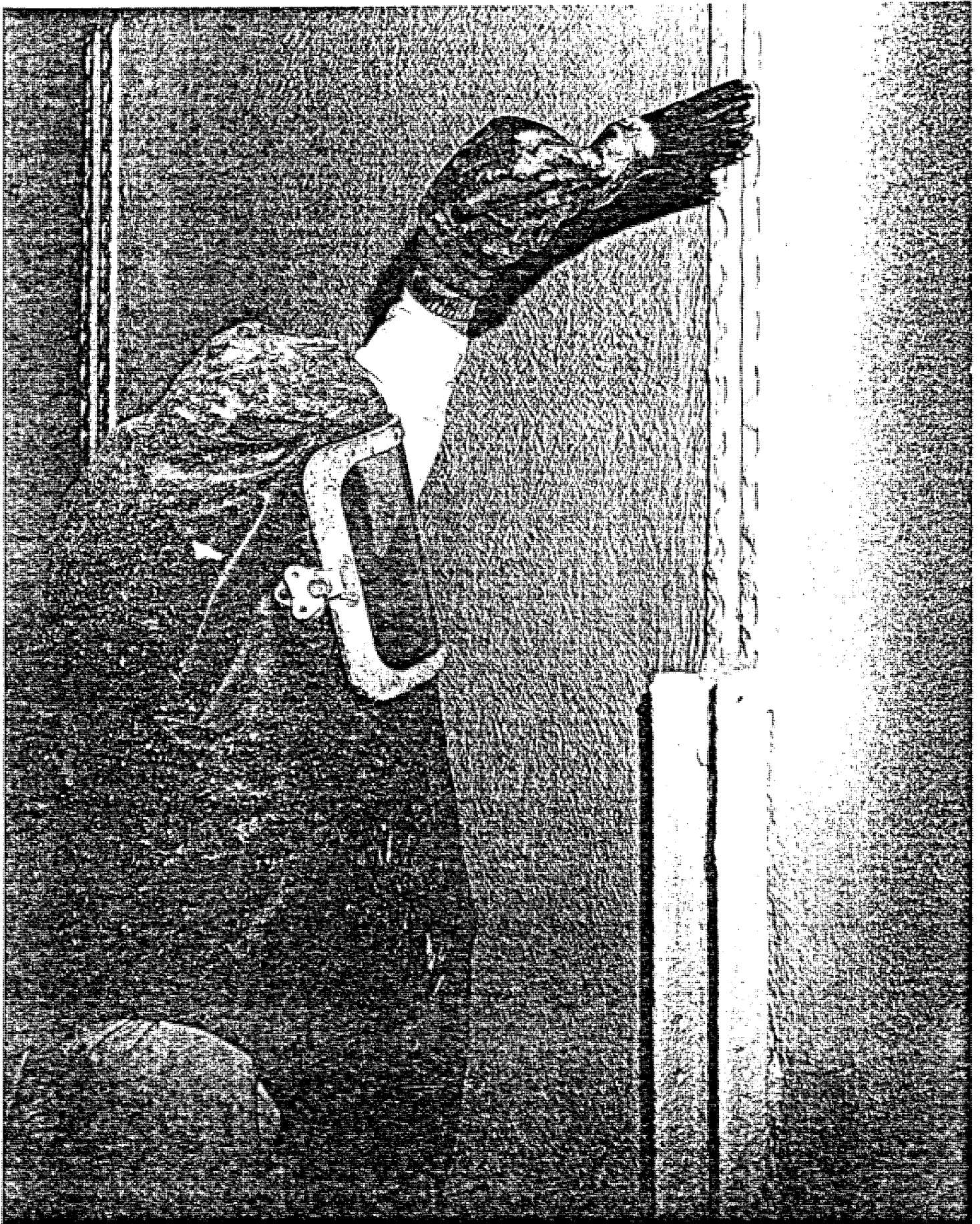
FIGURE 4-2. Application of Glassflake Type 202. Finish brushing to insure penetration into holes, etc. and to orient glassflakes in resin, thus providing laminar matrix and maximum resistance to vapor penetration and abrasion. (Photograph Courtesy of Glassflake International)
