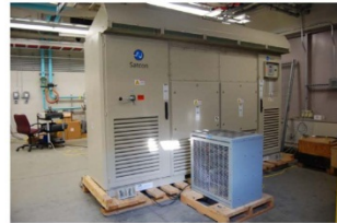
500 kW PV converter in FSU-CAPS lab
