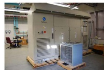
500 kW PV converter in FSU-CAPS lab
