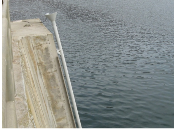
Figure 3.7. Trolley pipe mounted on a main pier of the John Day Dam powerhouse showing a cone used as a guide for trolley insertion.
